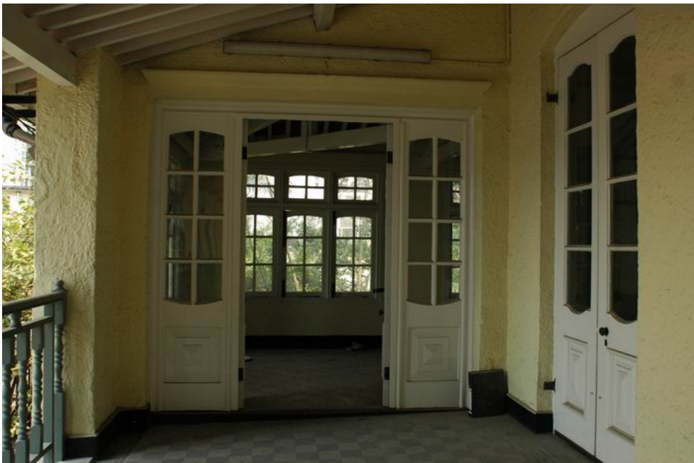
Fig. 455. Timber doors with segmental-headed glazing, opened to 1/F verandah of the main building.
