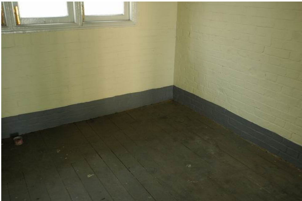
Fig. 457. Wooden planks flooring.
