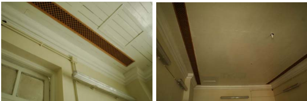
Fig. 458. Timber panelled ceiling with linear ventilation grills (linear grills were later improvement works).
