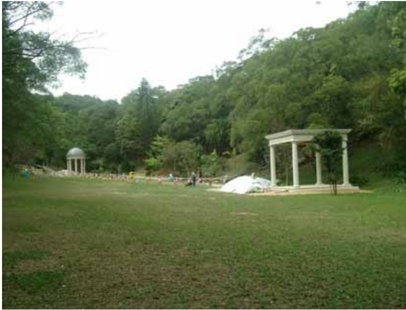
11. Open space behind the Gate Lodge with a rotunda, gazebo and pathway under construction
