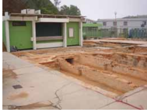
2. Site of the FML with exposed foundations looking towards the existing kiosk (Backfilled in March 2009)
