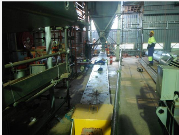
Dust Extraction Unit – ELB installing dust extraction unit screw conveyor on 48m level. Construction on 48m level is ahead of schedule.
