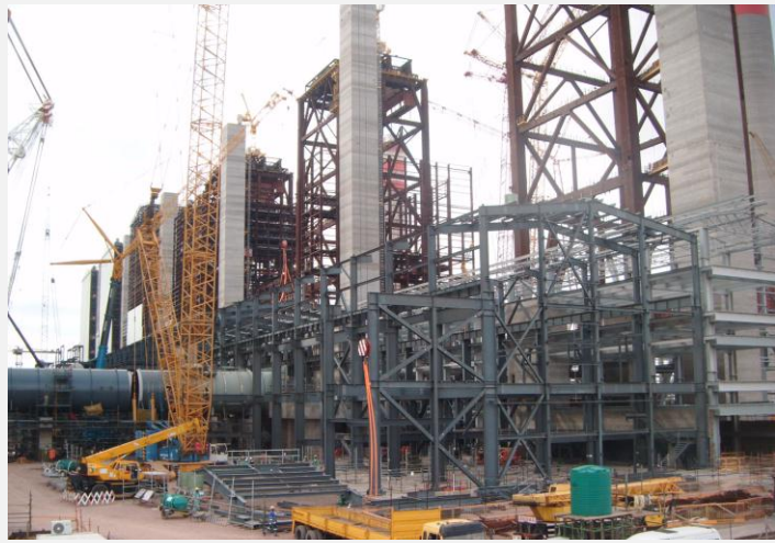
Unit 1 and 2 the Turbine Hall steel frame becomes on continues structure from North to South
