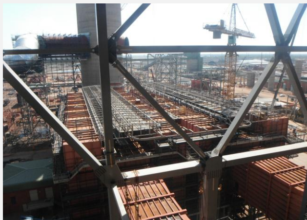
PJFFP Roof Structure – Very good progress is being achieved by DB Thermal
