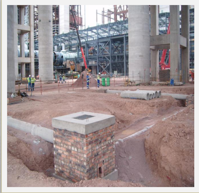
Unit 1 drainage works progress well following good access arrangements between MPS/JV and Alstom/Kentz
