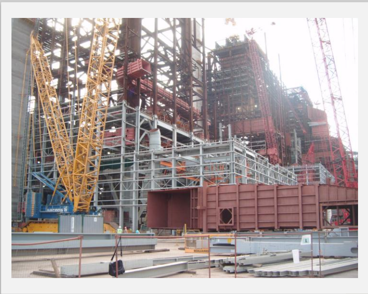
Unit 2 the 1200ton crane moves onto unit 2 and prepared to lift an 80ton section of ducting.
