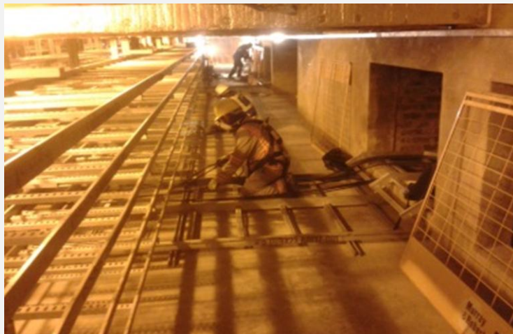
13.6m Cable Tunnel Strapping: Alstom P17 has started with their first cable pulling on the 21 st Oct 2014.
