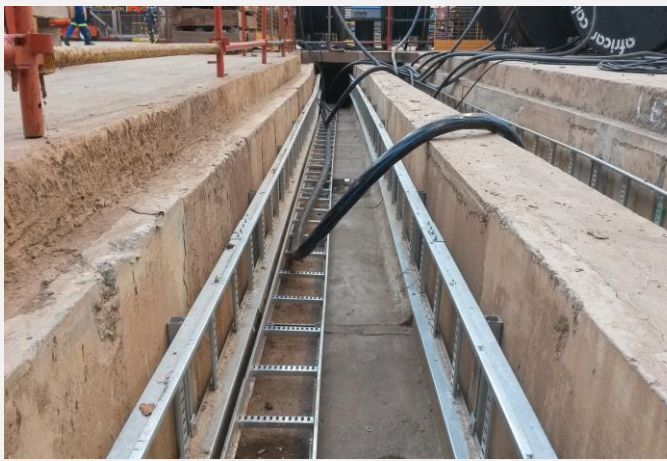
Installed and signed off cable racking to ID Fan motor terminal box. Installation of MV cabling in progress
