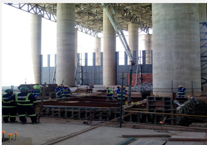
The final wind-cross foundation for Unit 5 has been cast along the loading bay access. This will ensure erection of all the wind crosses in order to be out of the way for back energizing (safety precaution)
