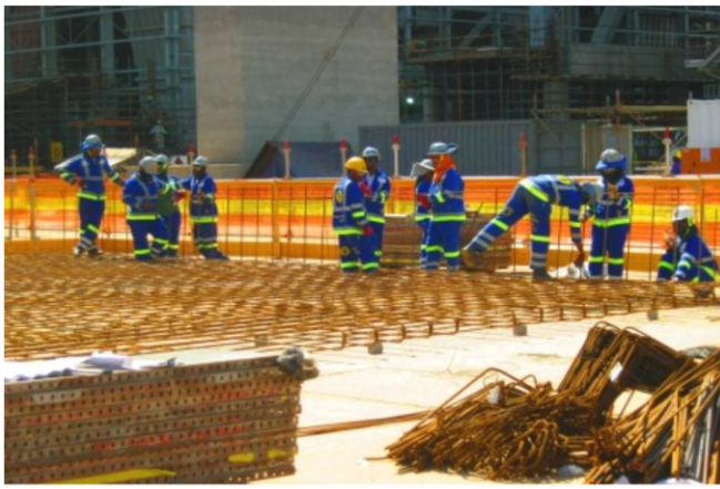
Pulse Jet Fabric Filter Plant (PJFF) substation building works have begun on Unit 3
