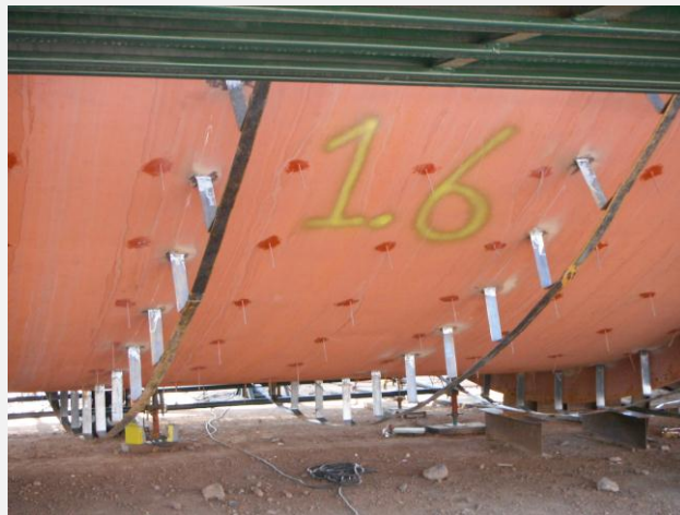
ID Fan to Chimney ducting – Component 1.1 – 1.10, completed installation of pinning and sub-structures.
