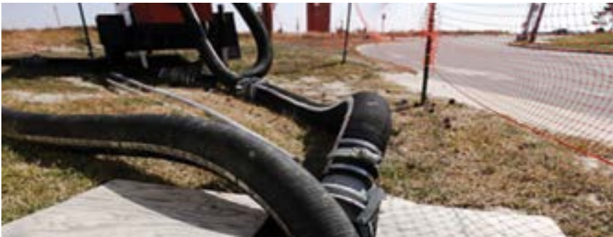
A temporary generator replaces a pump station damaged by Superstorm Sandy floodwaters.
