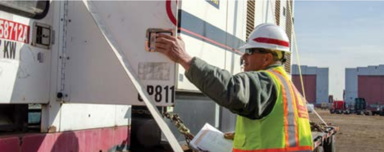
A U.S. Army Corps of Engineers' employee services a generator before it is returned to the warehouse. [Source: Liz Roll/FEMA.11/20/2012]
