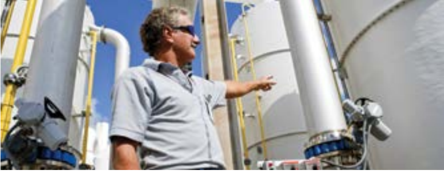
Water and Wastewater Plants Require a Large Quantity of Treatment Chemicals
