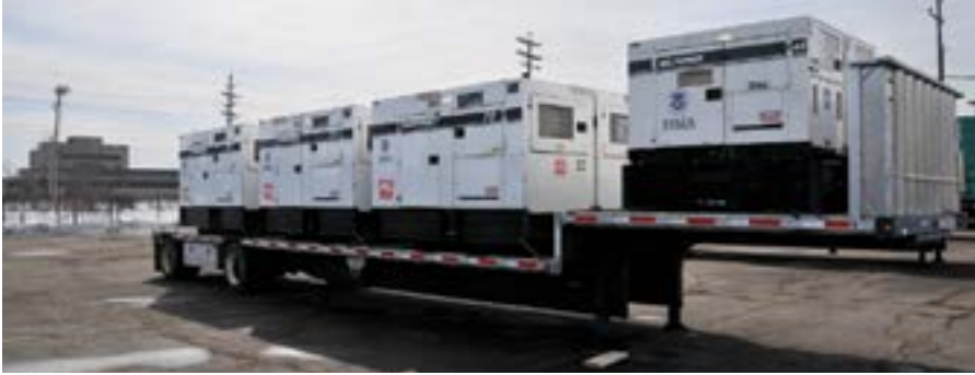
Emergency Power Supply Generators Staged at the Incident Support Base for possible use during Spring Flooding in the Midwest, Twin Cities Army Ammunition Plant, Arden Hills, MN. [Source: FEMA 03/18/2011]
