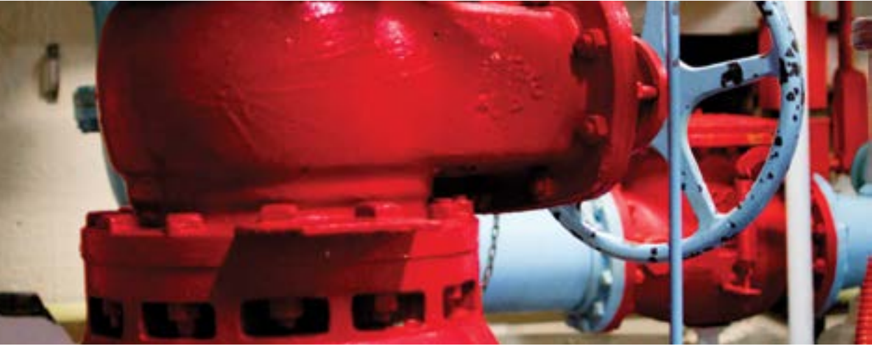
Valves at Water Plant
