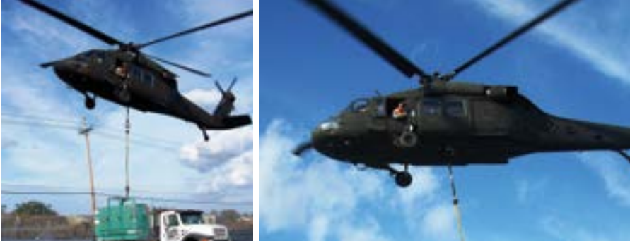
Members of the Memphis District Emergency Power Planning and Response Team airlift an emergency generator to place on top of a water storage tank at the Port Sulphur (Louisiana) Water Plant [Source: Photo by Memphis District]
