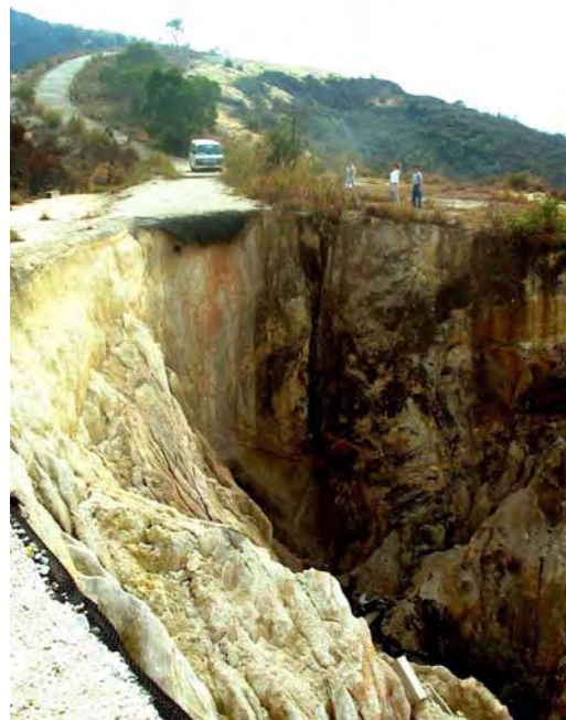
Gullies cutting across the road
