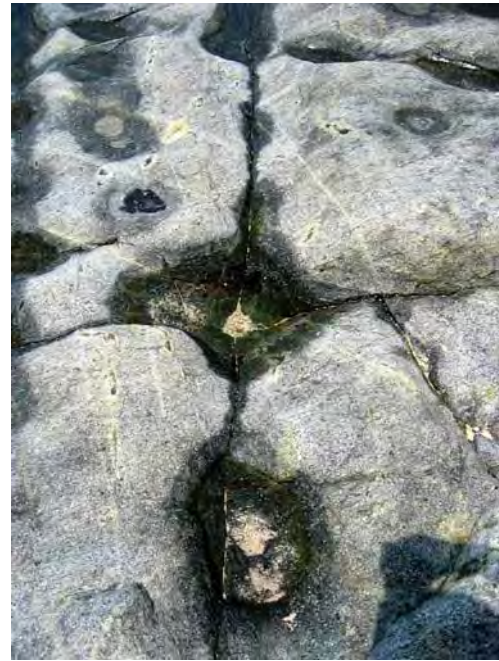
Erosion concentrated along joints
