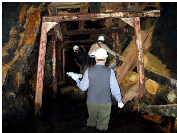
Abandoned mining tunnel in a dangerous condition
