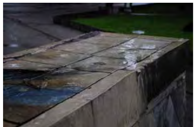
Fig. 3. Detail of the war memorial: Water ‘pooling’ on top of the artwork in the rain (Photo: R. Morelissen).
