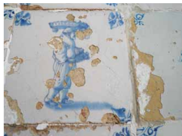
Fig. 6. An example of salt damage resulting in 'shivering' of the glaze (Photo: Kate van Lookeren Campagne).
