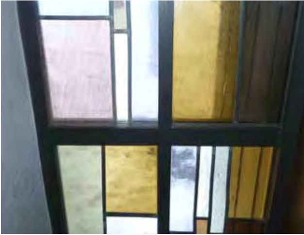
Fig. 4. Type of double-glazed protective glazing known as 'sandwich glazing', installed around 1990. Photo: authors.
