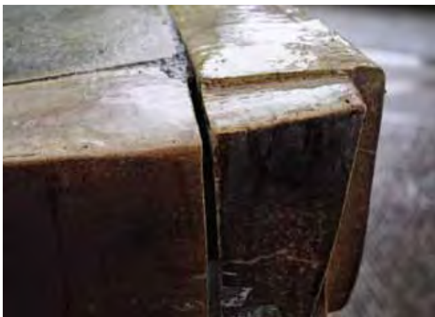
Fig. 6. Mortar-loss on top of the war memorial (Photo: R. Morelissen).
