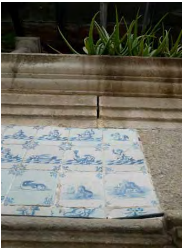
Fig. 8. The poor state of the grouting in the stone facade (Photo: Kate van Lookeren Campagne).
