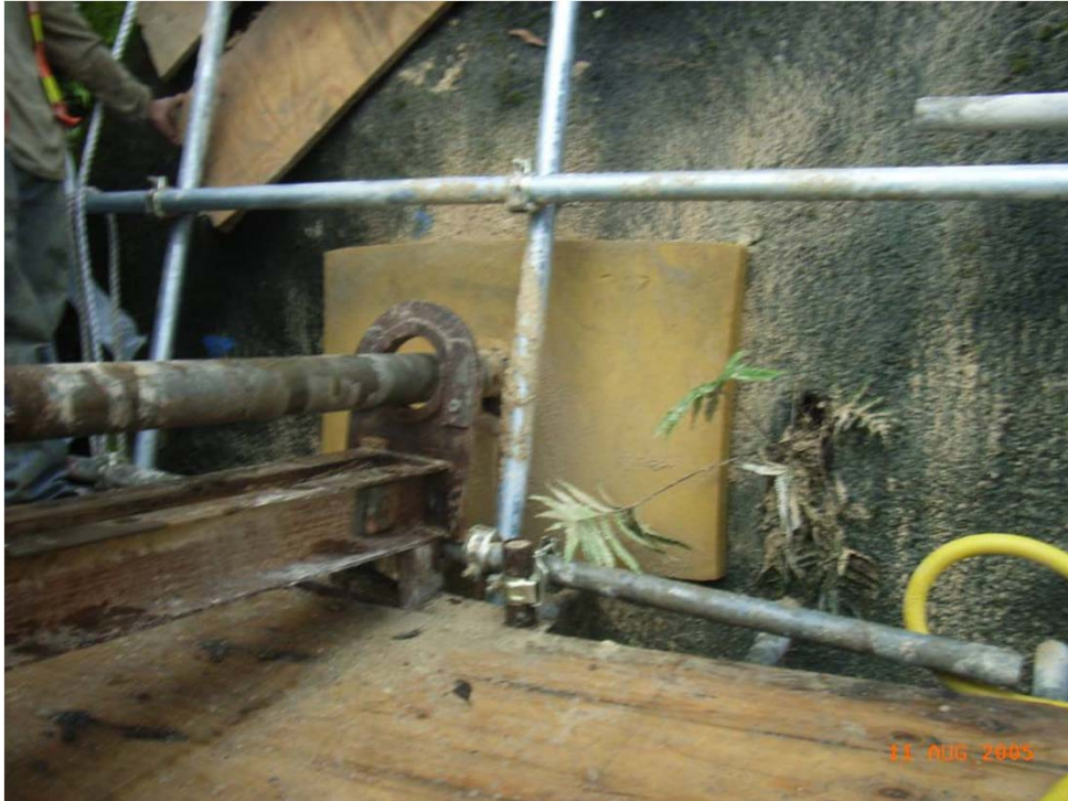
Photo 1 - A wet sponge should be placed on the slope surface to absorb most of the fine dust generated during drilling works
