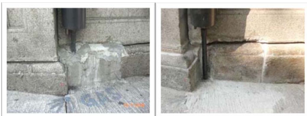
Photo 2.4 – Damaged portion previously patched with cement mortar
