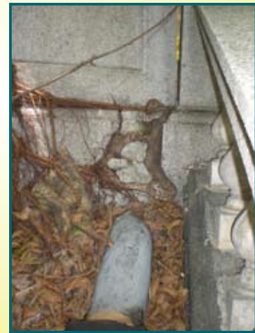
Roots from adjacent wall tree growing into joints of parapet wall and stone column
