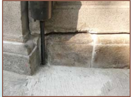
Damaged portion after repairing by specialist contractor
