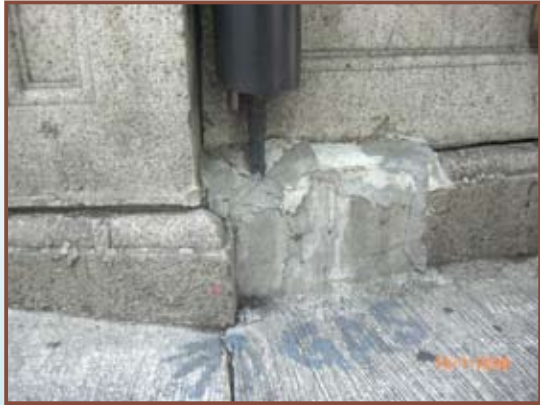
Damaged portion previously patched with cement mortar
