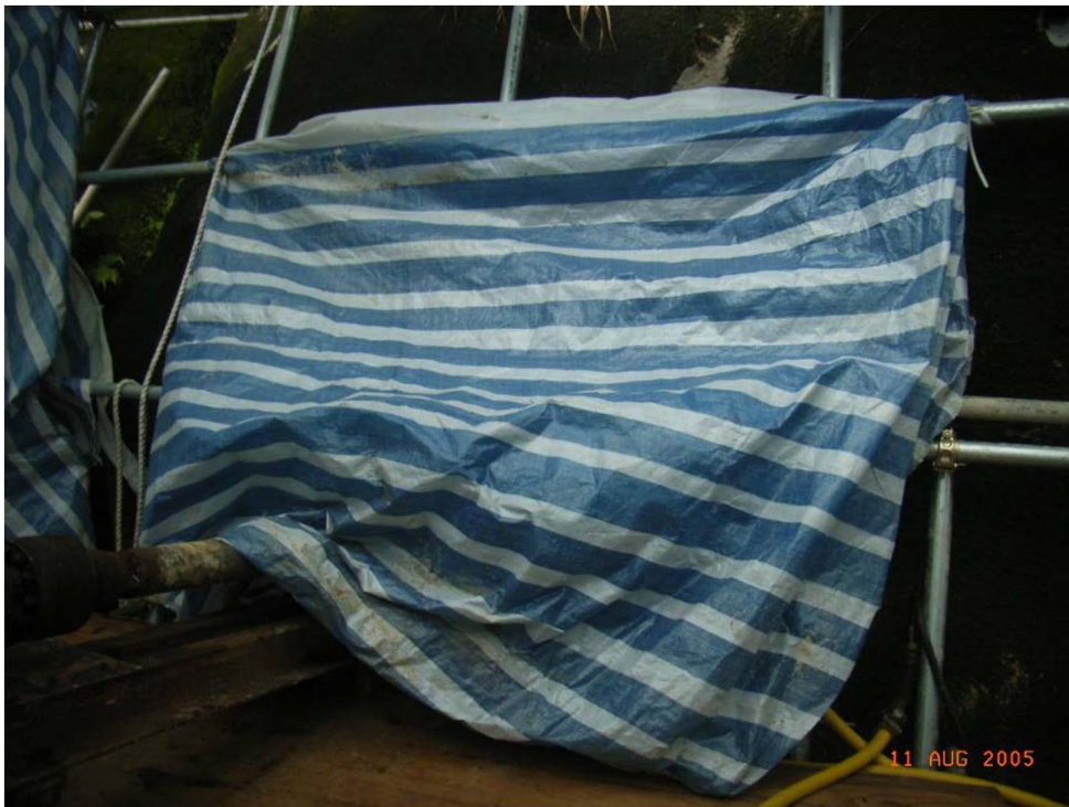
Photo 4 - Second layer of tarpaulin should be covering everything including the front portion of the drilling rig
