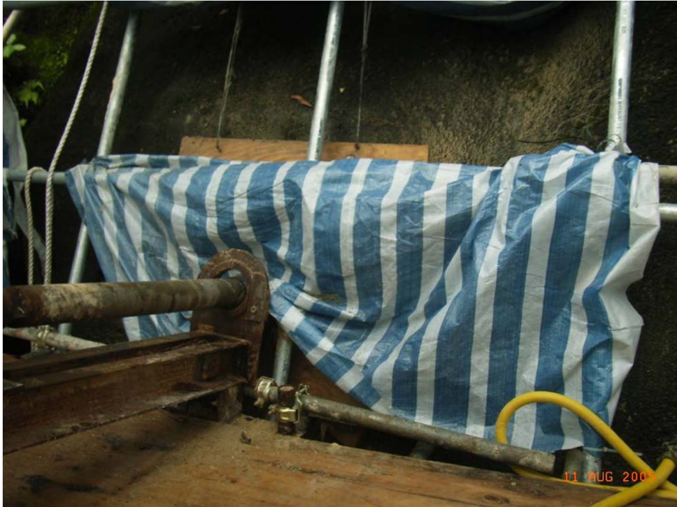
Photo 3 - First layer of tarpaulin should be placed above the sponge, the plywood and covering the opening of the drillhole
