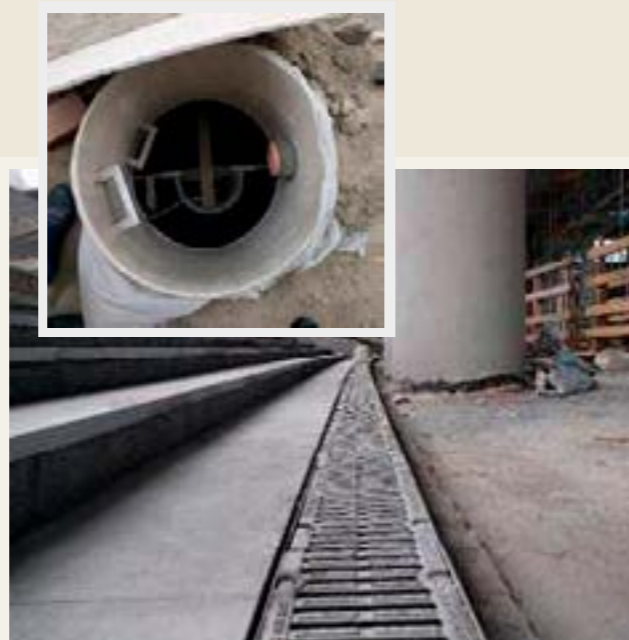
Fig. 34. Drainage system element and a grease trap
