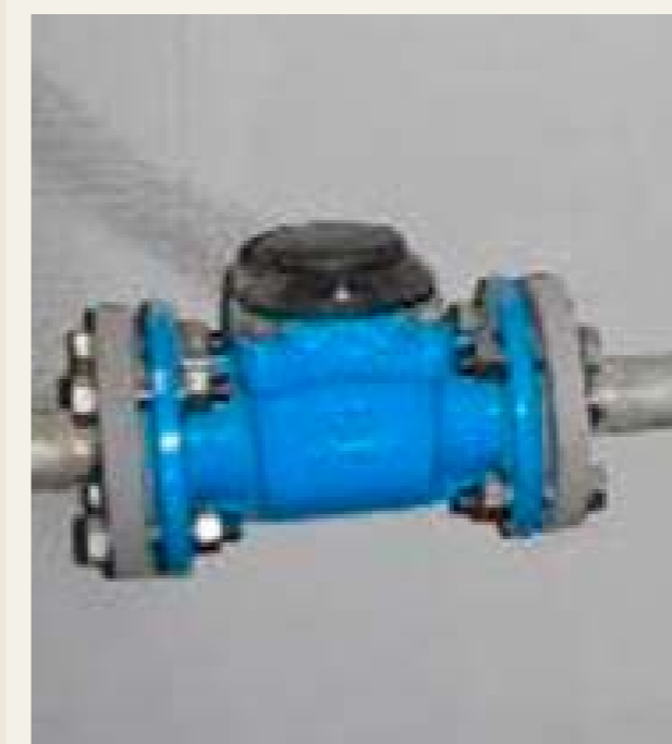
Fig.42. Water meter in Samara Arena
