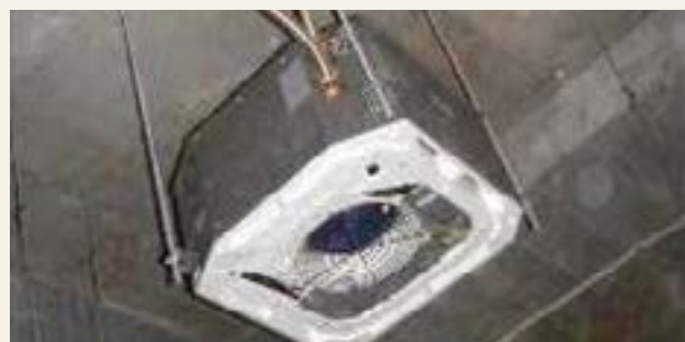
Fig.40. The installed fan-coil unit
