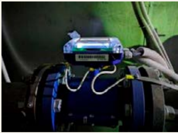
Fig. 33. Water meter in Volgograd Stadium
