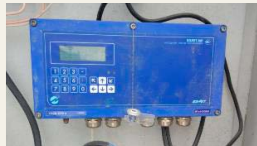
Fig. 23. Metering and computing complex in Rostov Arena
