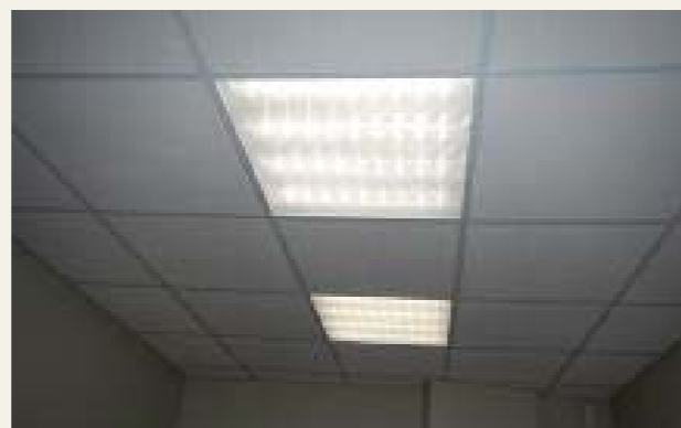
Fig.41. LED fixtures in the stadium
