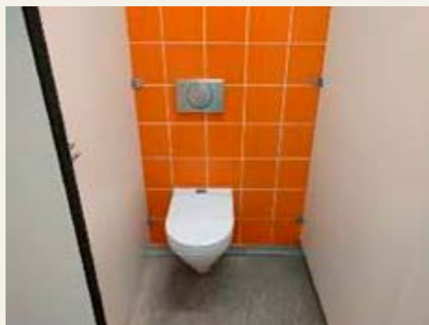
Fig.47. Toilet bowl and flush panel
