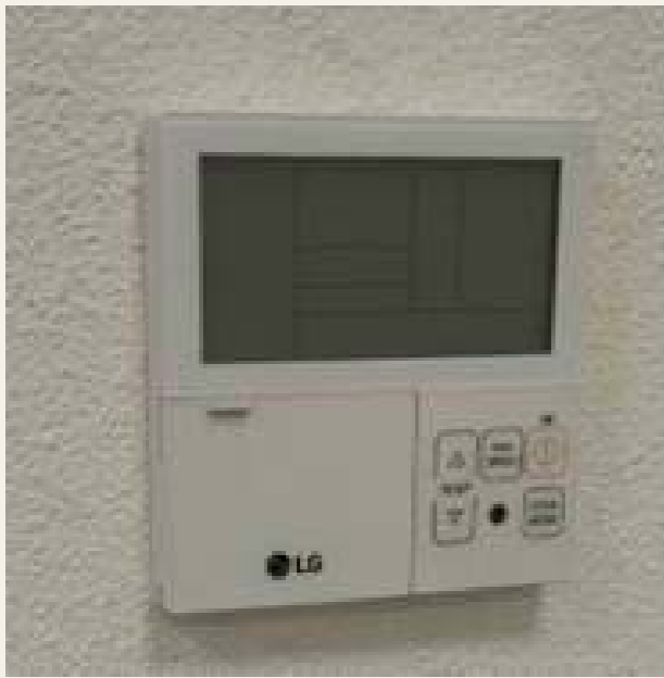
Fig. 21. Fan-coil unit control panel in Rostov Arena
