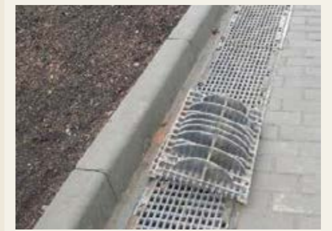
Fig.43. Water collection channels
