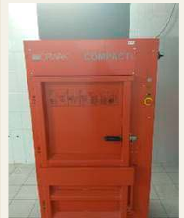
Fig. 17. Press compactor in Luzhniki Stadium
