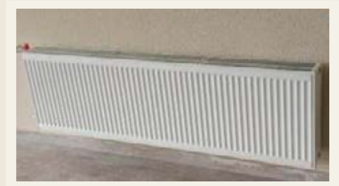
Fig. 4. Radiator with a thermostatic valve
