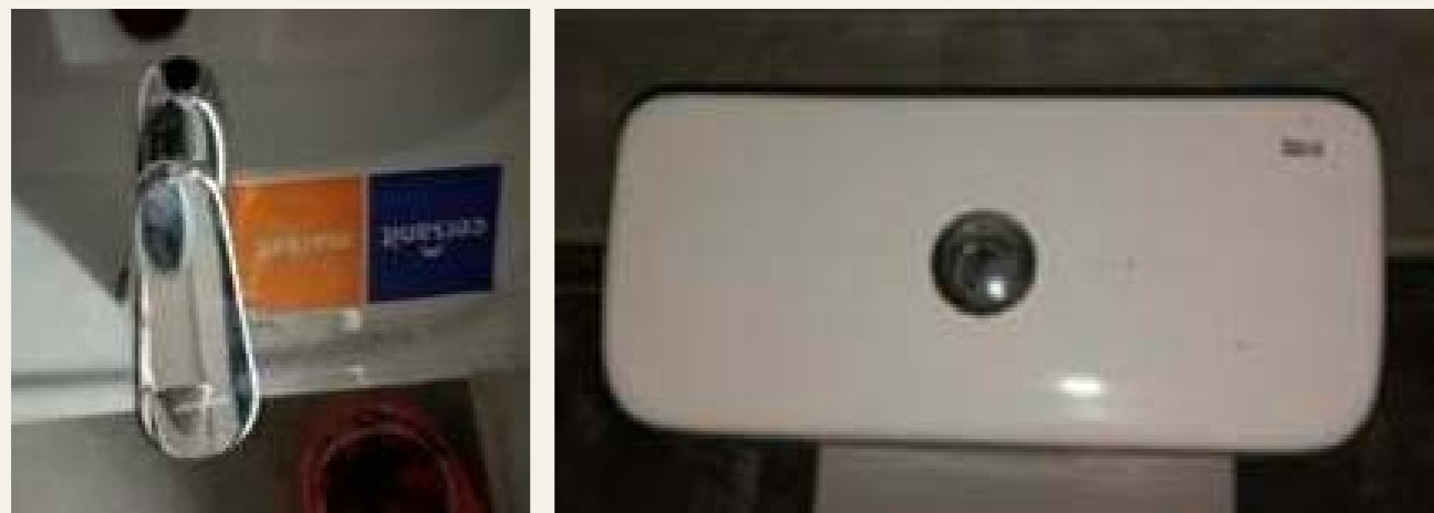
Fig. 5. Water-saving sanitary fittings in Kaliningrad Stadium
