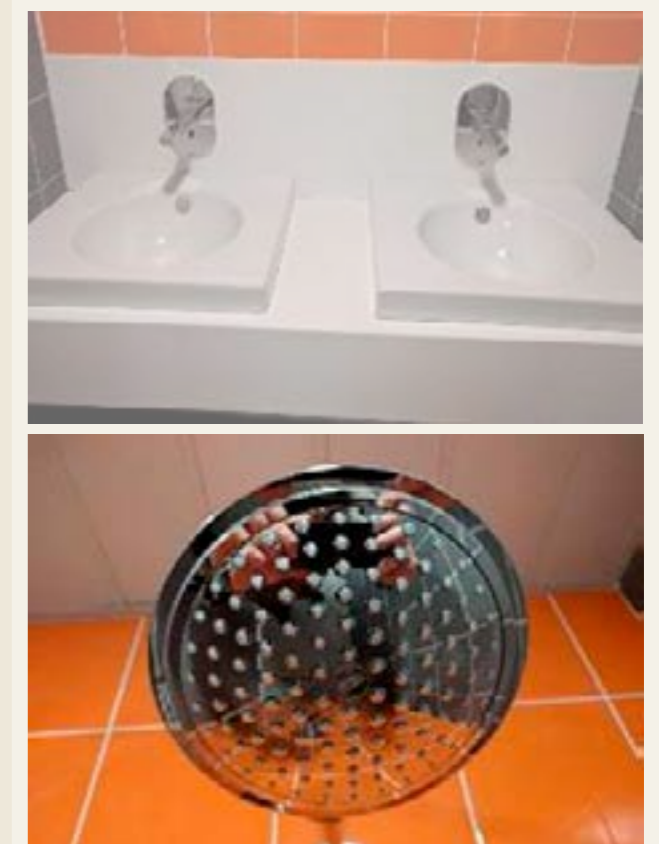
Fig.46. Taps and shower in Ekaterinburg Arena
