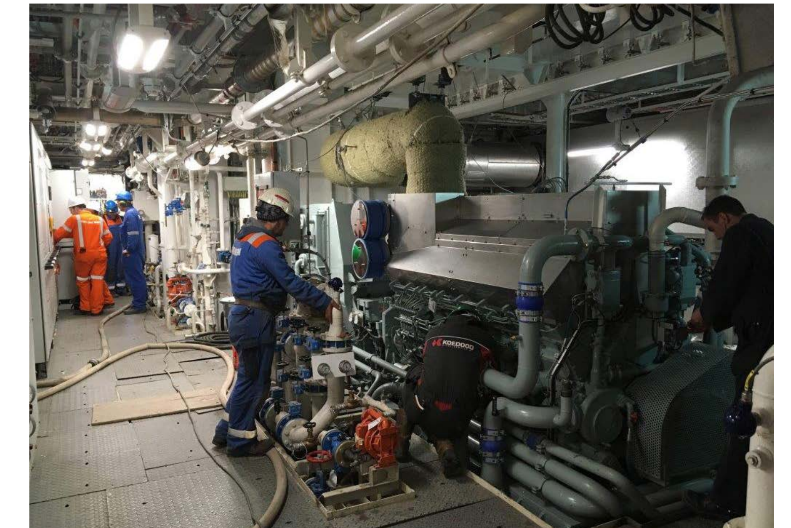
Getting the Engine Room Ready
