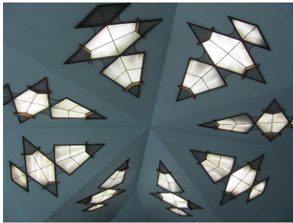
Figure 34: Main luminaires, Parow Oostersee Dutch Reformed Church, Conradie, 1973 in 2015. Photograph by the author.
