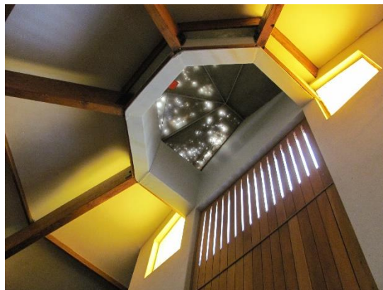
Figure 45: View of skylight, Constantia Dutch Reformed Church, Pelsler, 1973 in 2015. Photograph by the author.
