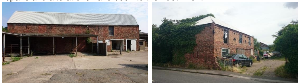
Figure 4.2: Agricultural buildings at Gibdyke Farm (left) and Northfield Farm (right), showing unsympathetic metal roofs, inappropriate alterations and in the case of the structure at Northfield Farm, visible structural defects.
