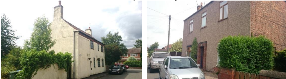
Figure 4.4: Here modern renders have covered over historic brickwork, masking historic architectural features (such as window arches and eaves corbelling) and harming local character. In the case of the property on Dame Lane (left), the render has been applied up to, but not over, the eaves corbelling, resulting in an awkward finish that clearly shows the building was not meant to be rendered. On the building on West Street (right), the pebbledash applied to the front gives the building the appearance of a mid-20 th century structure, but the brickwork on the side clearly identifies the buildings as late-18 th century. Changes to the openings and the addition of a brick door surround have exacerbated this harm.
