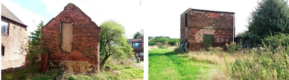
Figure 4.3: Former agricultural buildings on Top Street (left) and Gibdyke (right), both in a state of disrepair. The building on Top Street is unusual with its stone plinth facing the road, although its overall condition detracts from its significance. The structure at Gibdyke has also seen its original roof lost and other unsympathetic changes.
