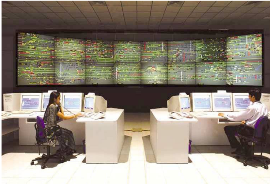
Train Management System at Mumbai
