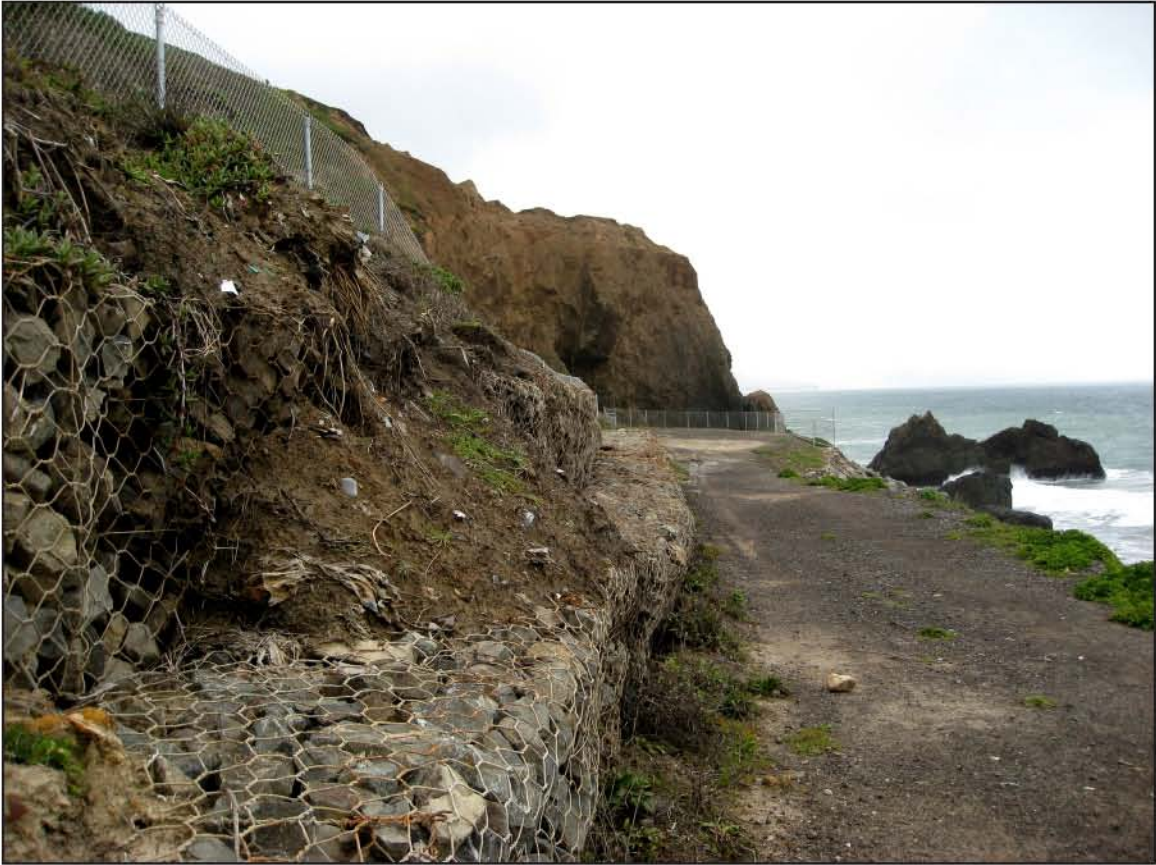
Figure 37. Three generations of seawall and riprap in gabions, stacked on top of one another, with slumping from the main landfill pit above. Photo by Shawn Heiser.
