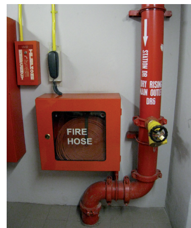
• Dry mains & standby fire hose
