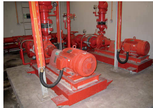
• Fire pumps for sprinklers
