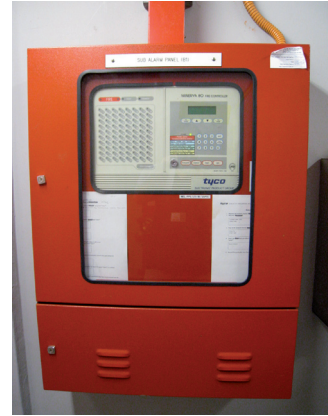
• Fire alarm panel
