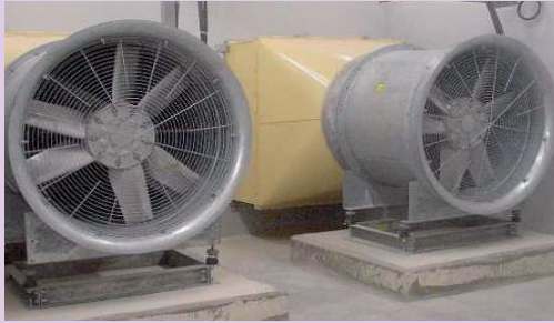
• Smoke extraction fans
