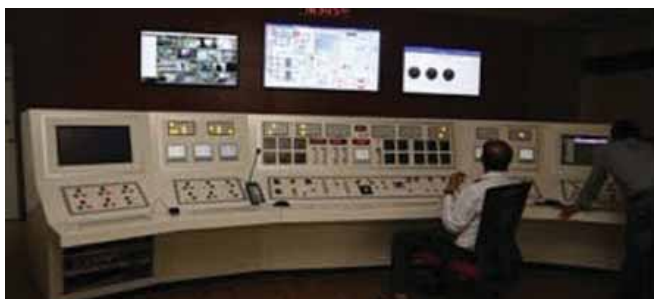
APSARA Control Room
