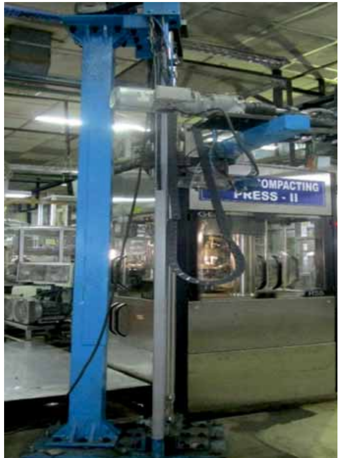
Rotary press transfer system
