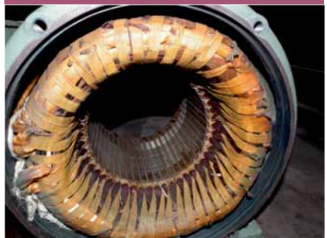
Moderator Pump Motor Stator Assembly after EQ Tests
