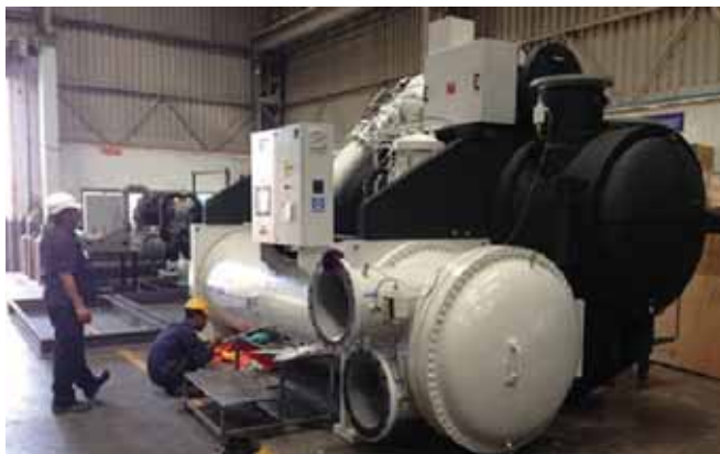
Largest capacity chillers ever made in India for ITER
