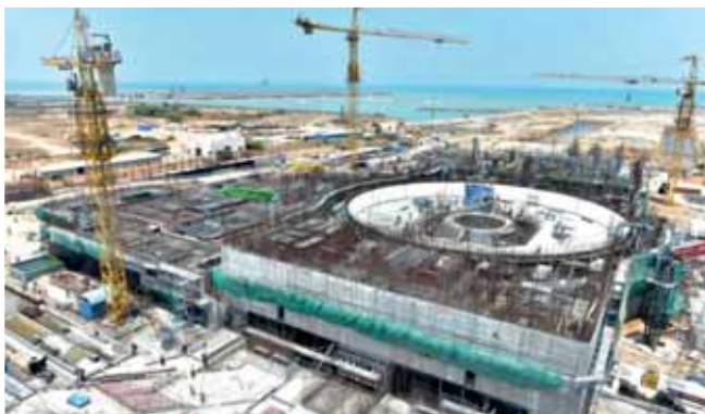
Kudankulam Nuclear Power Project (KKNPP) Unit-3&4
