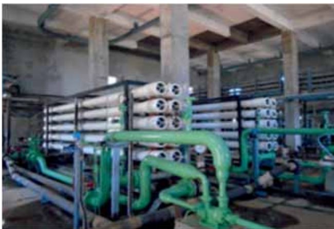
Desalination Plant at Zirconium Complex
