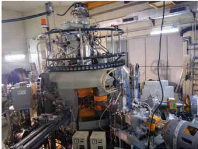
Cyclone-30 at Medical Cyclotron Facility, Chakgaria, Kolkata
