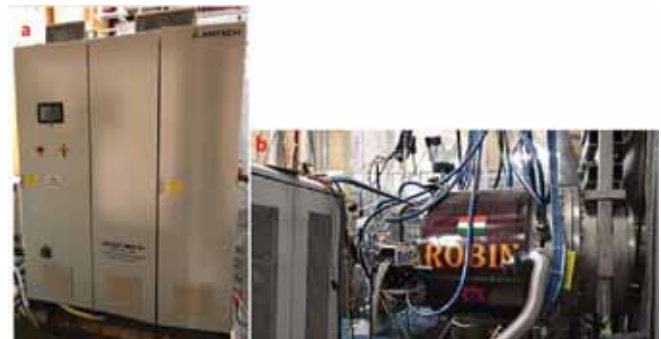
40 kW solid state RF generator (left) coupled to the negative ion RF ion source test bed (ROBIN) (right)
