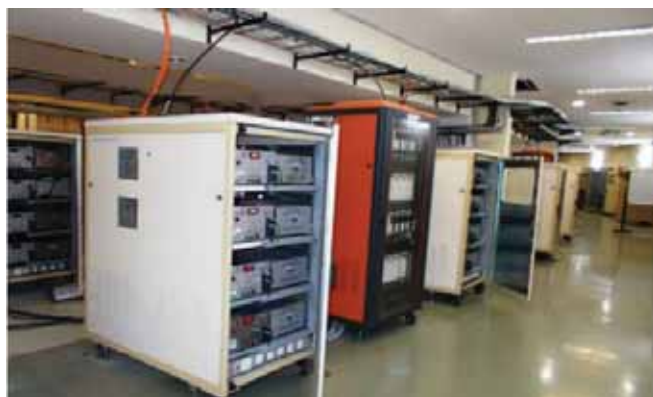
Active shunts commissioned in the power supply hall of Indus-2
