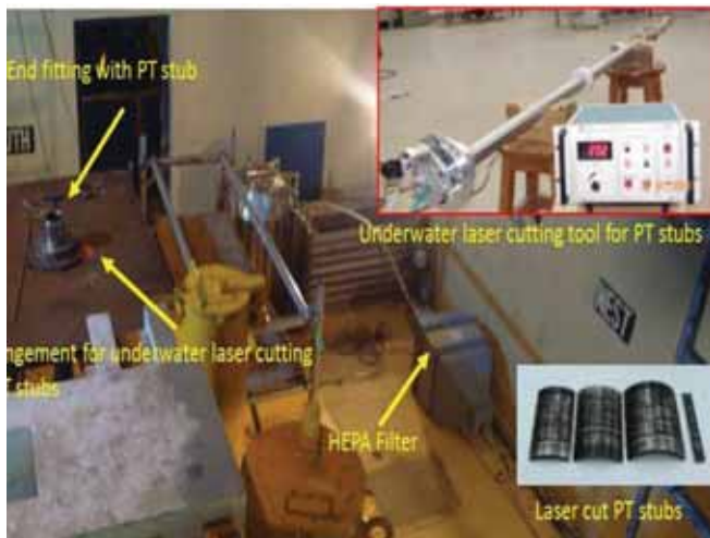
Underwater laser cutting arrangement for PT stubs at MAPS-1 (Insets show laser cutting tool for PT stub and laser cut PT stubs)
