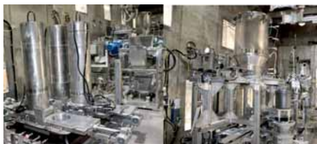
Process equipments erected inside containment Box of PPRDF
