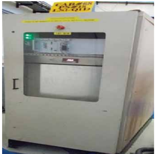
The installed and operational power converter for LS1Q1D magnet in Indus-2
