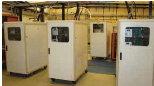
FOFB Power Supplies installed in the power supply hall of Indus-2
