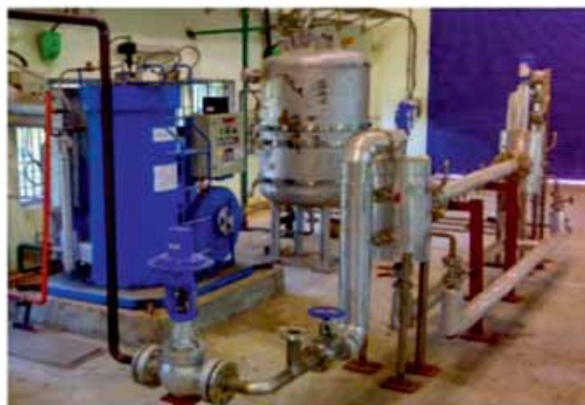
Water and Steam Interaction Facility (WASIF) at SRI, Kalpakkam
