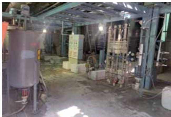
Gallium extraction facility at TDP, Mumbai
