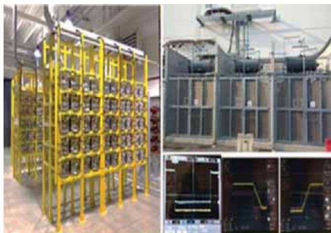
7.2MW, 100kV Power supply at RFX, Padova, Italy
