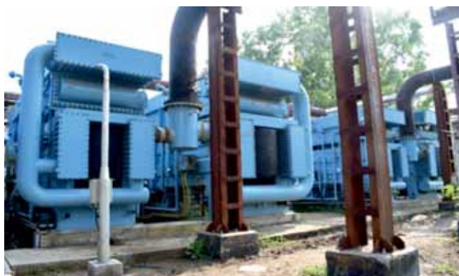
Hot Water Vapour Absorption Refrigeration (VAR) machines commissioned at HWP, Manuguru
