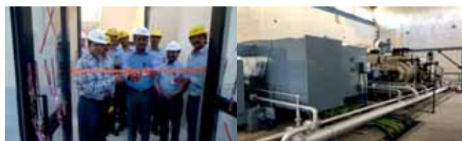
Chief Executive, HWB inaugurating test operation of Steam Turbine Generators (STG) at HWP, Kota
