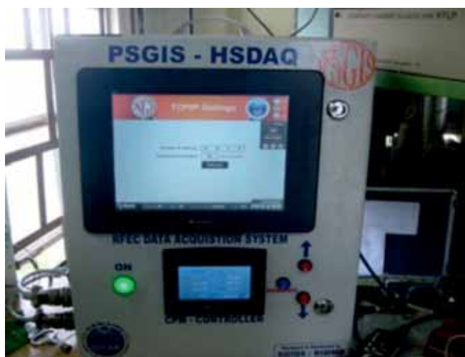
HSDAQ - HMI control panel
