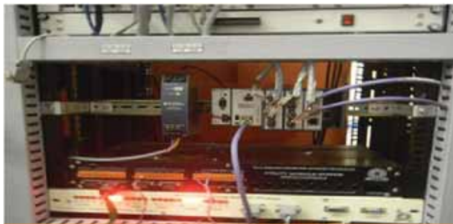
Distributed fast data acquisition module installed in Indus-2 MPS hall
