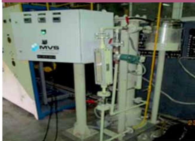
Commissioning of Gas Humidifier System in Sintering Furnaces
