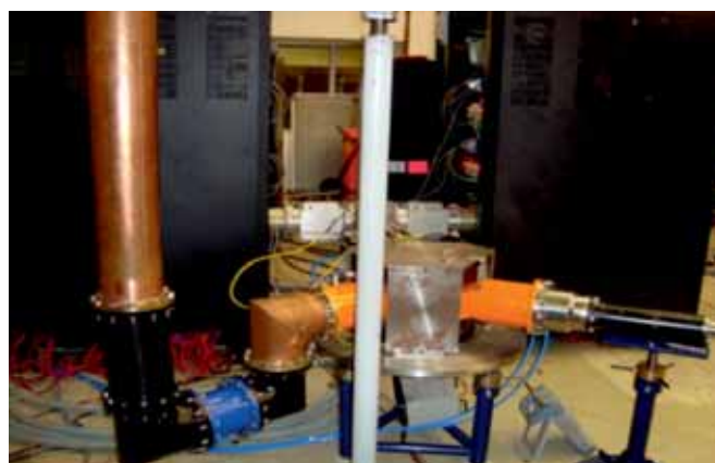
View of installed RF circulator at Sixth Indus-2 RF station
