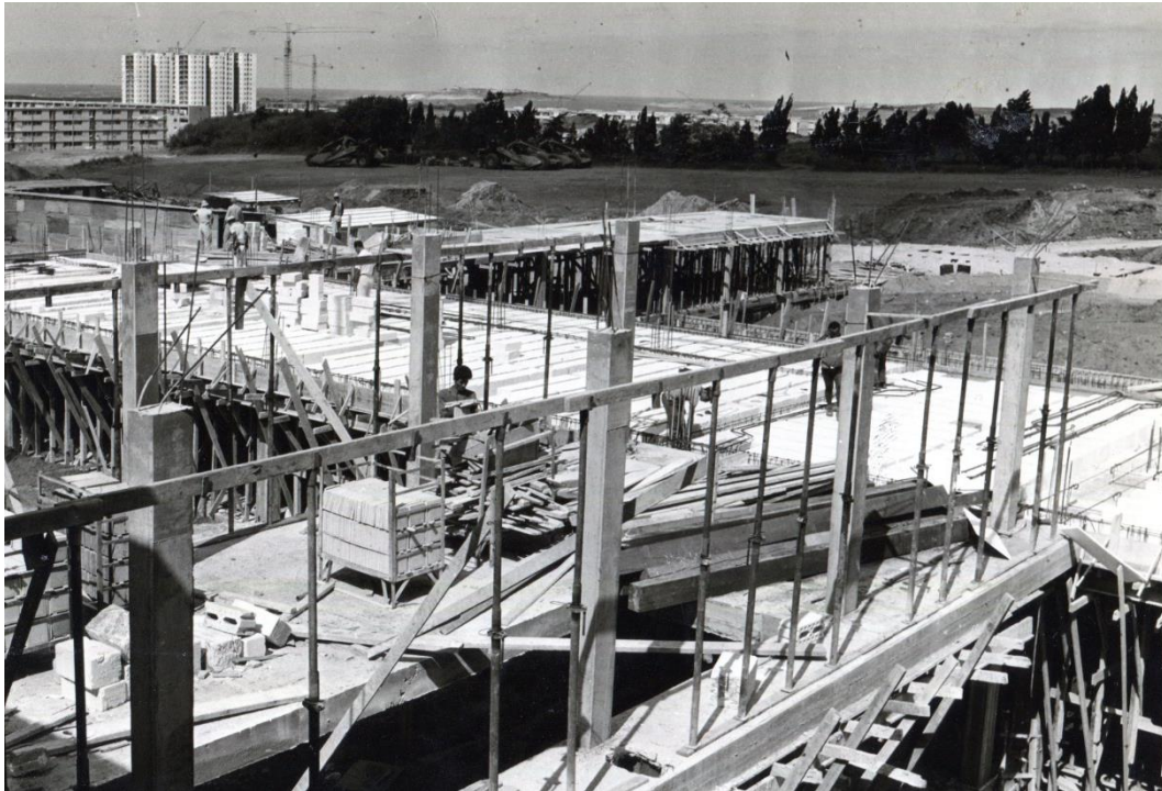
Figure 4.47: Gilman Building, laying Ytong blocks for the casting of the ceiling above the basement of the northern wing, 1964 (photograph by Isaac Berez, Tel Aviv University Archive)
