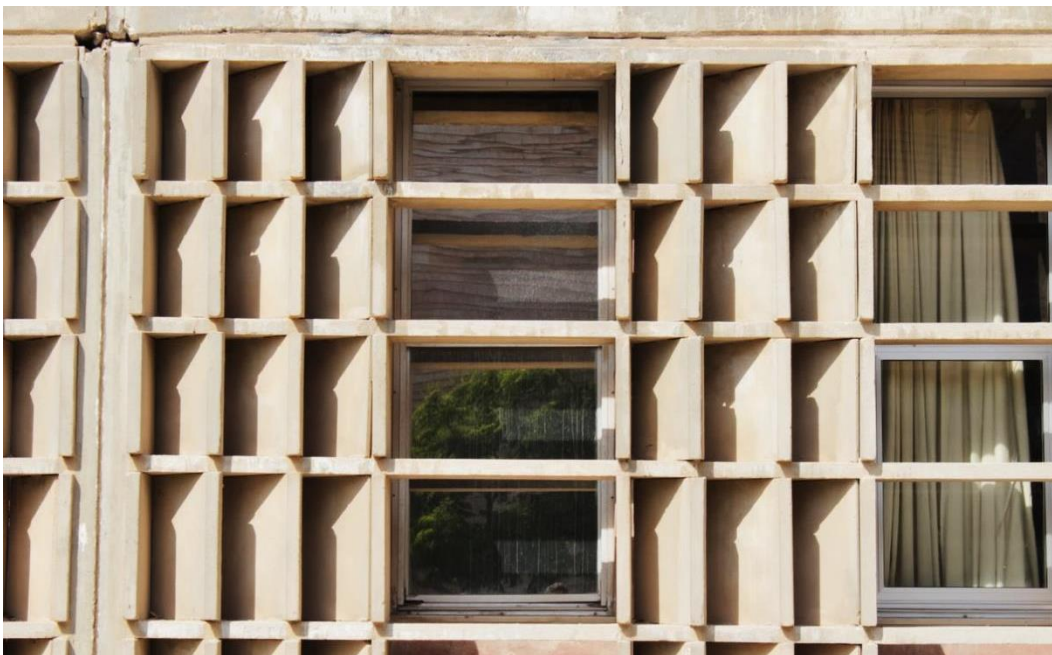
Figure 4.36: Gilman Building, the concrete sun breakers of the eastern facade of the northern wing, 2012 (photograph by the author)
