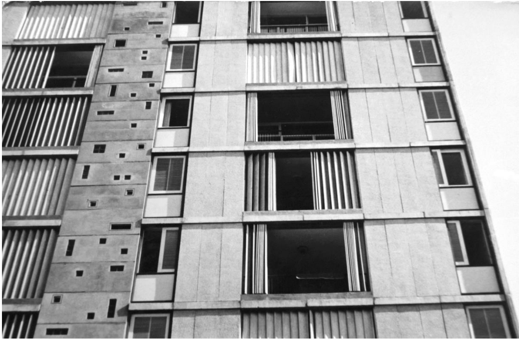
Figure 4.25: Nahum Zolotov, 79 Ben Yehuda Street, Tel Aviv, 1958, the western facade showing the Trisol shutters in their full operational range between total closure and total openness. The facade's windows received sliding wooden shutters with rotatable slats. Photograph by Nahum Zolotov (Nahum Zolotov Collection, Information Center for Israeli Art, The Israel Museum)
