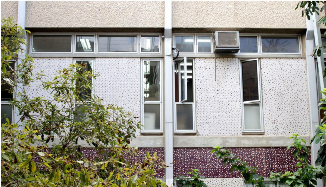
Figure 4.48: Gilman Building, the southern wall of the northern courtyard (northern wing) showing external coolant pipes running from air handling units on the roof and an old window air-conditioner, 2012 (photograph by the author)
