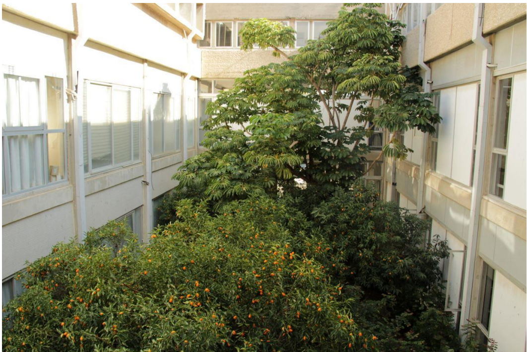
Figure 4.44: Gilman Building, the smaller courtyard of the southern wing, looking east, 2014 (photograph by the author). The original PVC-aluminium shutters were replaced during the 1970's with opaque panels made out of asbestos cement and metal, combined with narrow windows
