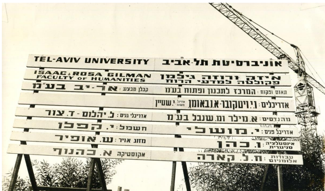
Figure 4.2: The official sign at the Gilman Building construction site indicating the names of the general contractor, architects, and engineers. Photograph by Isaac Berez (Tel Aviv University Archive). Stein's name appears (in Hebrew) next to the names of Wittkower and Baumann, with the title "junior architect"
