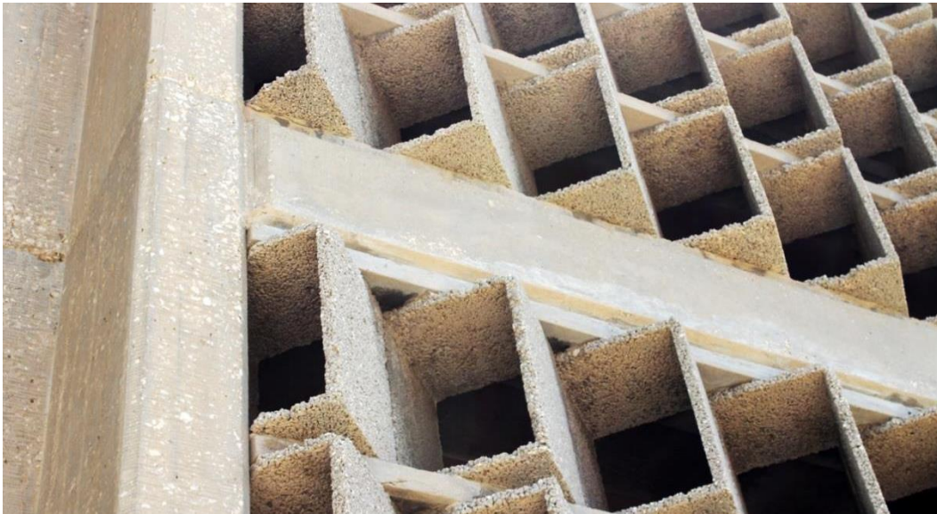
Figure 4.35: Gilman Building, the concrete sun breakers of the western facade of the southern wing, 2012 (photograph by the author)
