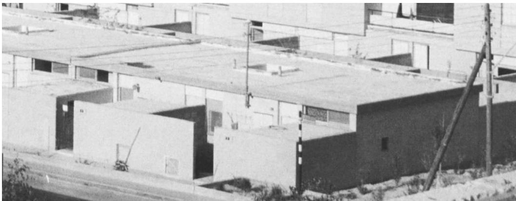
Figure 5.27: Carpet housing (house types B and D), a photograph from the mid-1960's showing the traces of asphalt on the inner side of the roof parapet (Rotbard 2007, 596)
