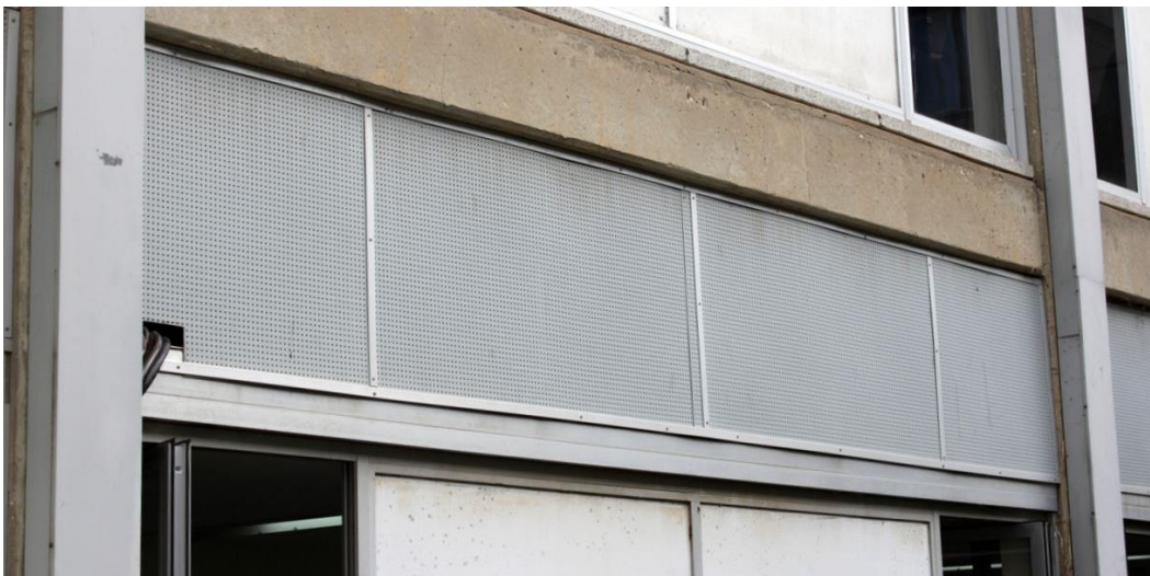
Figure 4.50: Gilman Buildings, a detail of a corridor wall facing the northern courtyard of the northern wing, 2012 (photograph by the author). The area above the recessed ceiling of the corridor was closed with perforated metal sheets upon the replacement of the original sliding shutters
