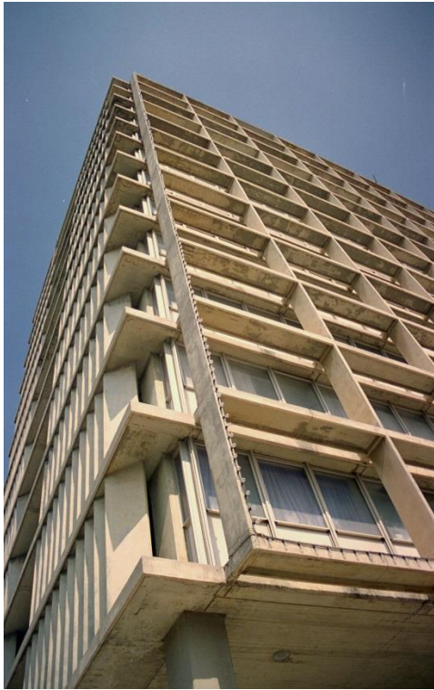
Figure 4.39: Menachem Cohen, the south-western corner of Tel Aviv City Hall (1957-1965), showing the "egg crate" shading array for the southern facade and the vertical shading elements for the western facade, 2001 (photograph by the author). The original shading elements of the southern facade were replaced during a recent renovation of the building by a new construction which unsuccessfully tried to mimic the original design
