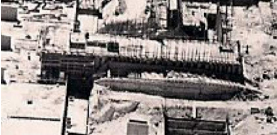
Figure 6.21: A detail from an aerial photograph taken during the construction of the main building of the university, showing the realized north-western facade of the basement floors of the Eshkol Tower, including the diagonal vertical sun breakers (University of Haifa Archive)
