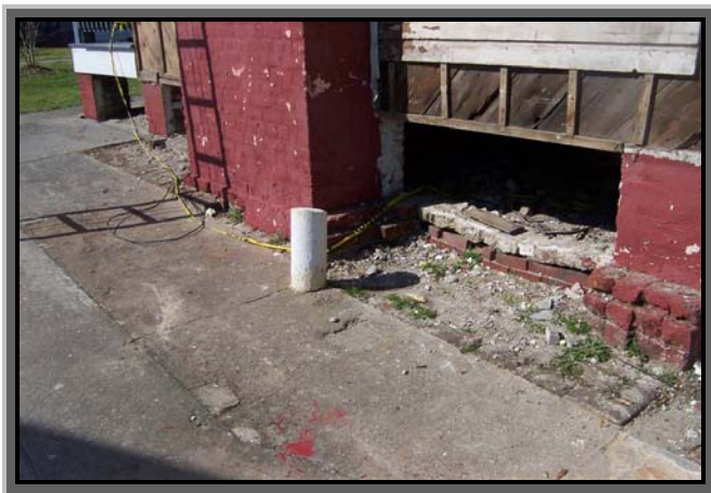
Figure 21. Southwestern View of Assistant Keeper's Residence, Showing Brick Foundation Just West of the Cement Walkway.
