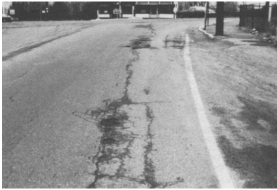
Moisture lying in pavement leads to raveling type of potholes
