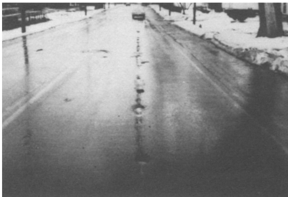
Longitudinal joint needs routing and filling
