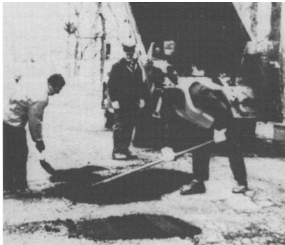
Patch potholes promptly
