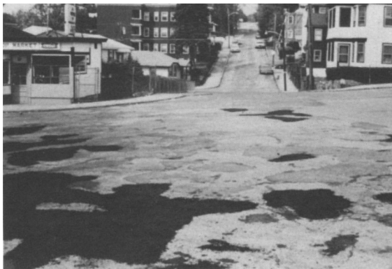
Pothole problem at intersections
