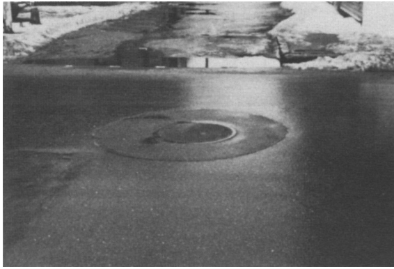
Repair should extend for about 5 feet in a square or circular area around manhole (a large enough area to remove stressed asphalt pavement)
