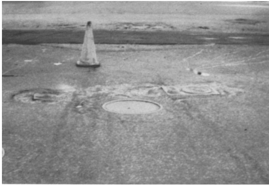
On thicker pavements surface raveling can be corrected by removing or reworking the top 1 in. as shown
