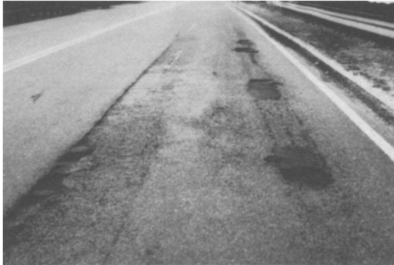
Severe case of poor density that led to raveling failure
