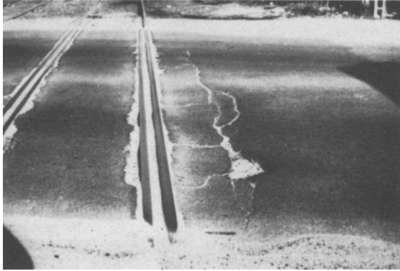
If ties are moving potholes occur at end of ties
