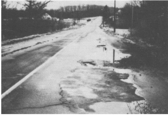
Poor shoulder maintenance traps water on road
