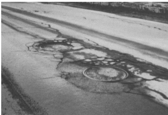
Utilities add to municipalities' maintenance problems
