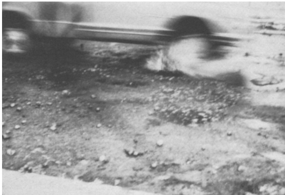
Emergency patches frequently fail
