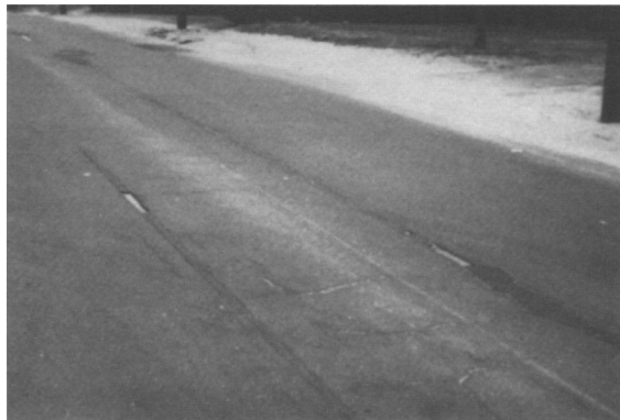
Overlay too thin to cover trolley tracks adequately.
