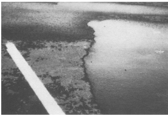
Surface water flows into cracks
