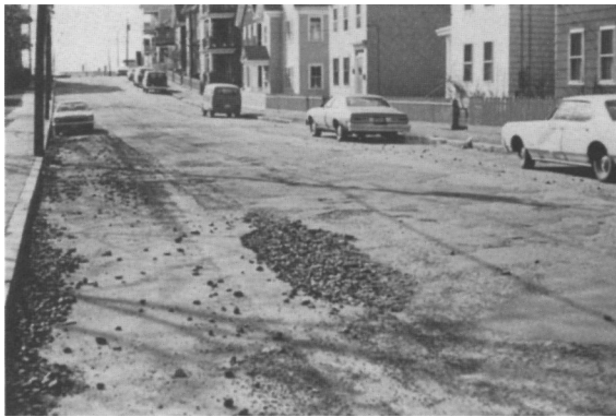
Macadam pavement unravels dramatically when water enters
