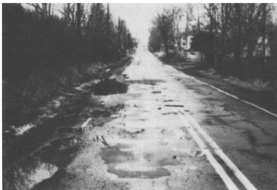
Example of the results of poor drainage
