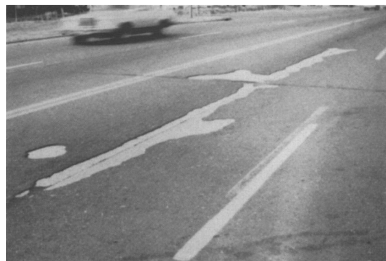
Delamination of thin overlay
