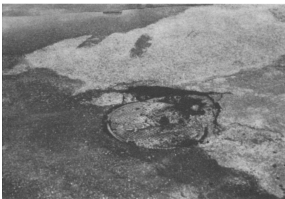
Breakout at manhole is most severe on thin pavements
