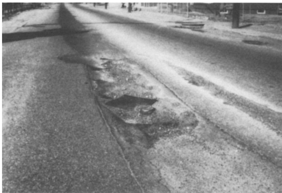
Failing utility trench patch
