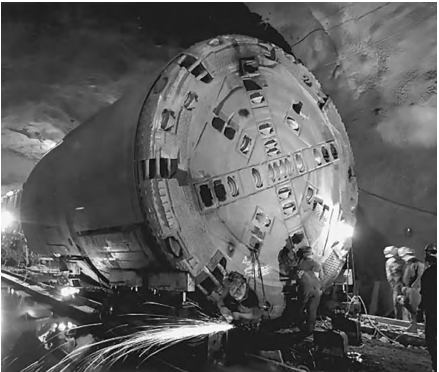
Readying Bore-Regard, the tunnel boring machine, to drill into the west hills during construction of Westside MAX, 1994
