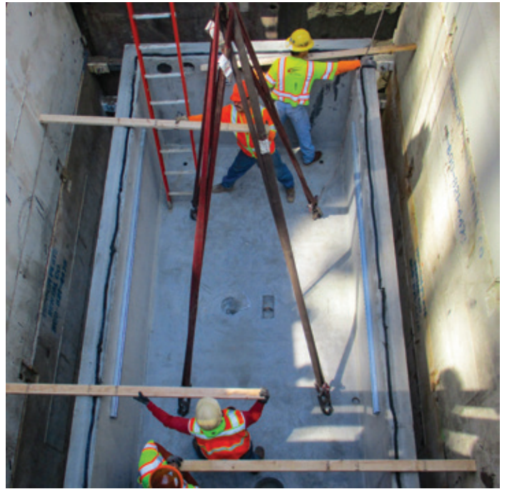
A utility vault is an underground room that provides workers access to utility equipment for maintenance. The image shows Metro contractors installing the new utility vault under the street surface.
