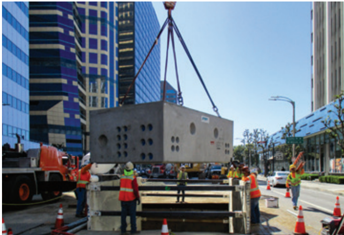
Before station construction can begin, numerous utilities that run under Wilshire Bl, such as water, power and telecommunications, need to be relocated so that service continues while the subway is being built. The image shows Metro contractors lowering a new utility vault into the ground on Wilshire Bl near Westwood Bl.
