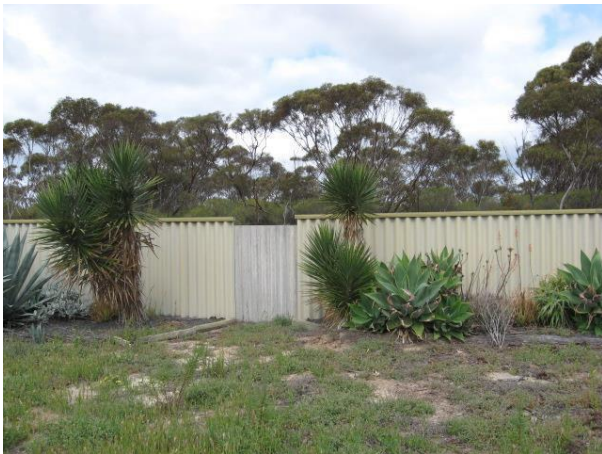
House 4; fibrous asbestos fence (to be removed)
