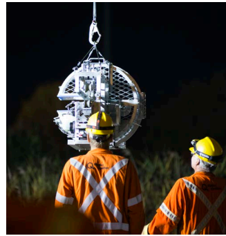
In the first phase of a broader deployment, anti-icing spiral rods were installed on transmission lines crossing major intersections in the cities of Québec and Lévis. The spiral rods prevent ice accumulation on high-voltage line conductors during use of the de-icing system at Lévis substation.
