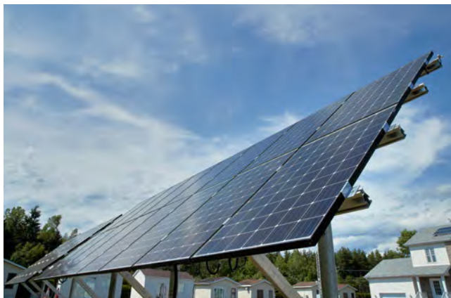
As shown by these solar panels at the LTE, we're studying various aspects of customer on-site generation using renewables.
