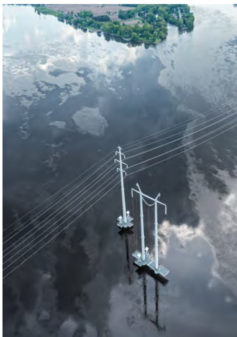
A line in the Chamouchouane–Bout-de-l’Île project at the Rivière des Prairies crossing in northeast Montréal.
