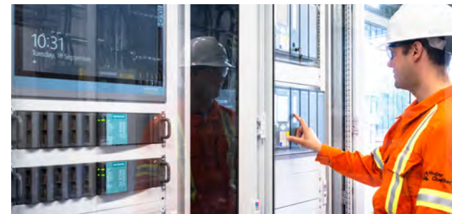
Tests conducted at Saint-Chrysostome substation in connection with a demonstration project for deployment of new digital technologies.
