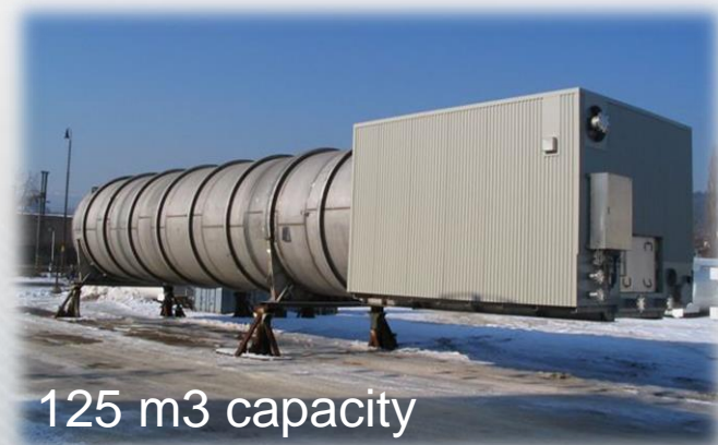
Fuel tank with „gas tight box“
