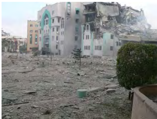
The science faculty building of the Islamic University in Gaza after the Israeli Air Force strike during Operation Cast Lead (Izz al-Din al-Qassam Brigades website, December 31, 2009).
