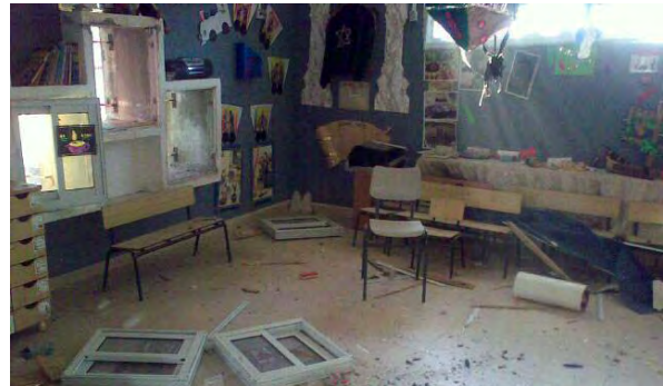
Damage caused to a kindergarten in Ashdod by a rocket hit (Photo by Yossi Landau, used courtesy of the ZAKA spokesman, January 6, 2009).
