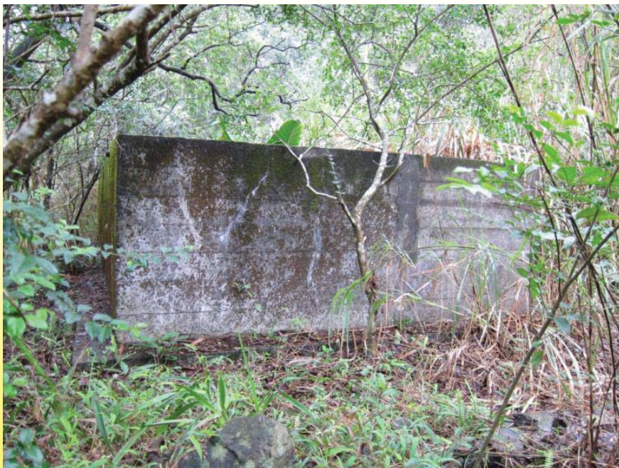
儲水池 Water Tank (1)
