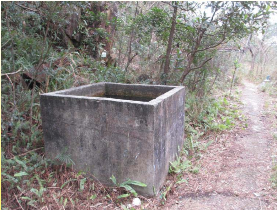
儲水池 Water Tank (2)
