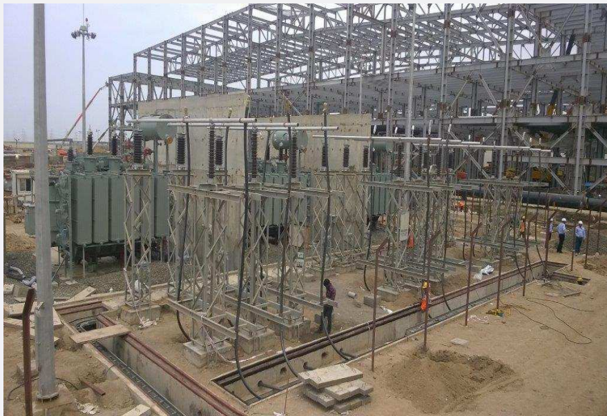
Pic 3: Transformer Yard
