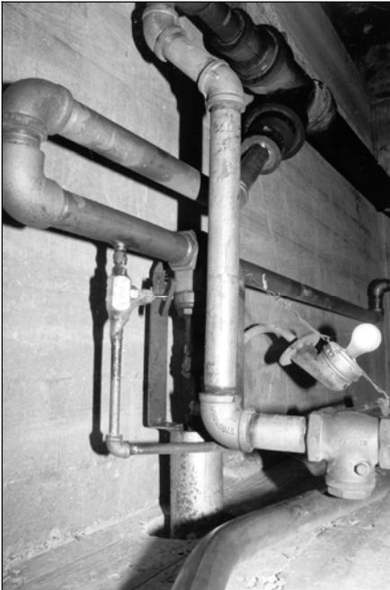
Fig. 94: Portion of plumbing and sewage system connecting chemical room to gas chamber.
