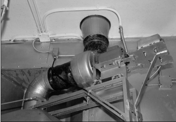
Fig. 88: Exhaust fan and stack on top of gas chamber.
