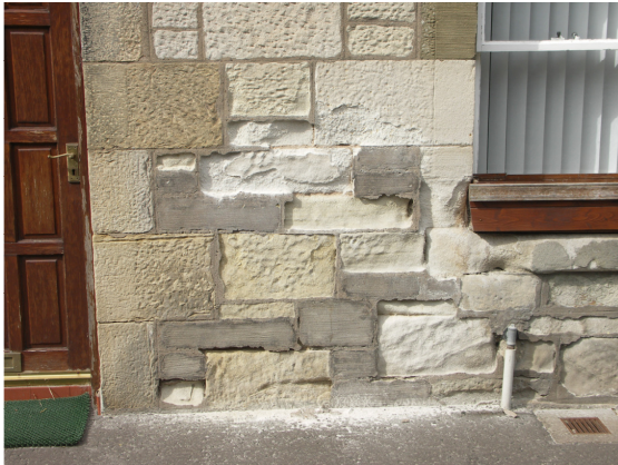
Mortar repairs in cement will damage sandstone masonry
