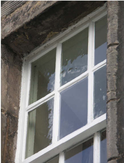
Modern plate glass does not match the original crown glass, while the white gloss paint is inappropriate.
