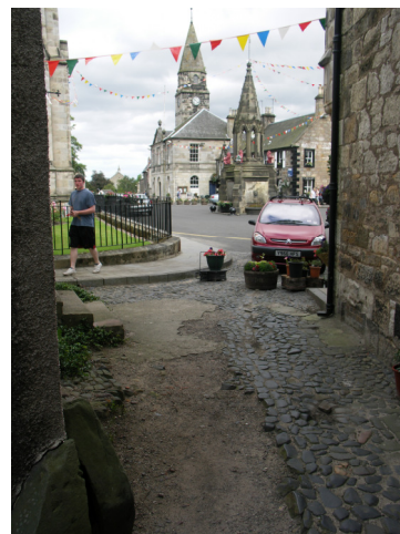
An old cobbled pavement in poor state of repair
