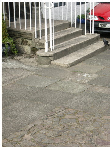
Cement re-surfacing of stone steps erodes townscape character
