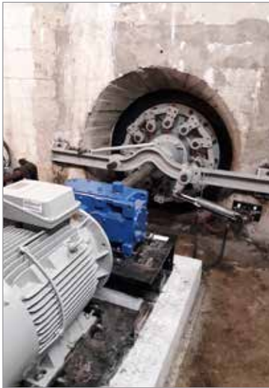
3 (top). Chris Elliot of On Stream Energy with the large turbine after restoration
