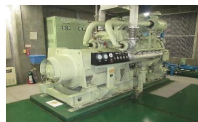
Procurement of Fixed private power generator
