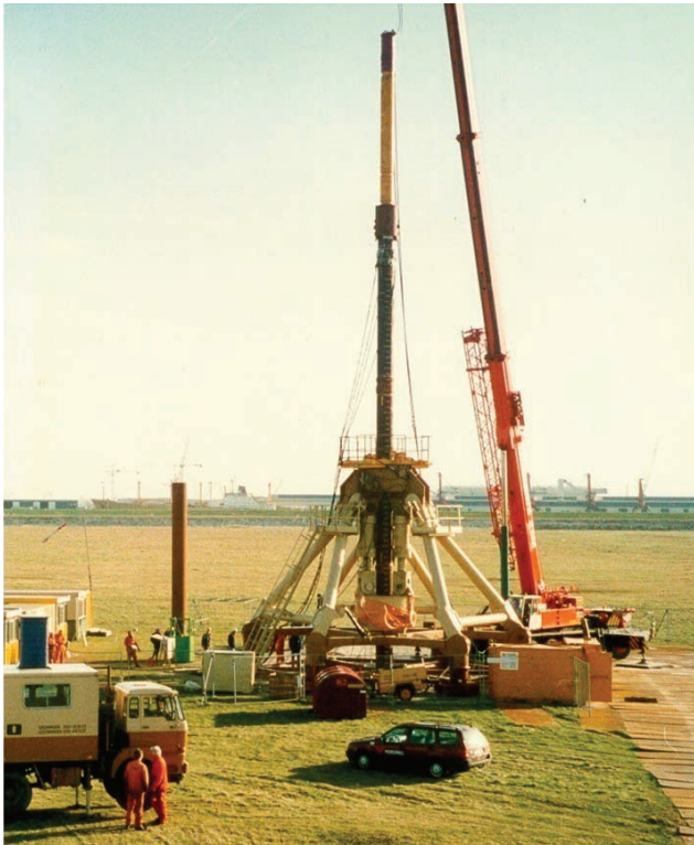
[FIG. 3] Pile driving at the Euripides site (photo courtesy Fugro Engineers B.V.)
