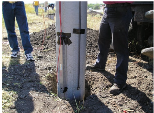
[FIG. 3] Strain gages and telltales attached at the toe of a pile.
