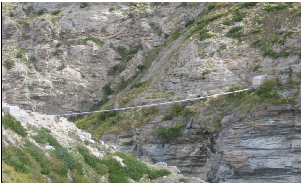
Figure 2.12: FES built water pipe suspended across Gaanka River to serve Milam Village
