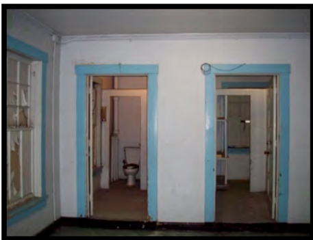
Figure 66: If toilet rooms on second level are to be used, the doorways need to be 3'-0" wide, if not the doors shall be replaced or new accessible toilet room shall be constructed on first level.
