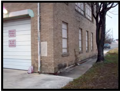
Figure 58: Sidewalk must be reconstructed to allow free access without any changes in levels due to land shifts.
