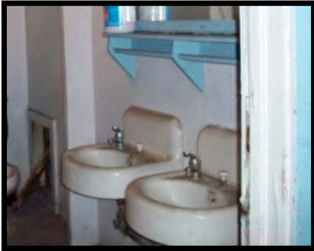
Figure 68: If sinks are to remain and made operable, they shall have a height of 34" AFF to rim. If sink is to be operable with hot water, then exposed pipes shall be covered with insulation and faucets shall be replaced with push-type.
