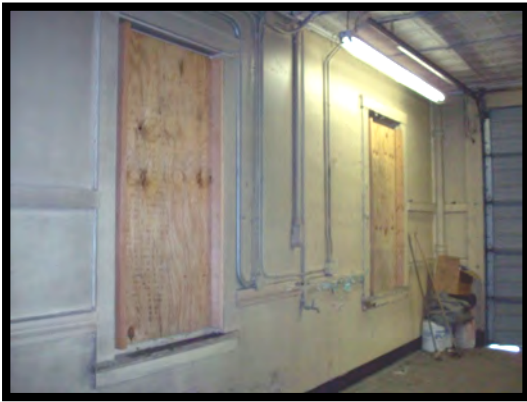
Figure 85: Provide high performance glazing or remove paint and plywood from existing windows to maximize interior day lighting.
