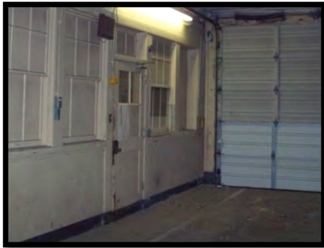
Figure 63: Doors on first level shall have new hardware that does not require twisting of the wrist if it is to be used as a major passageway. It is recommended that a panic device be used for easy exit.
