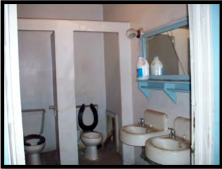
Figure 67: New soap and paper towel dispensers shall be provided no higher than 42" AFF.
