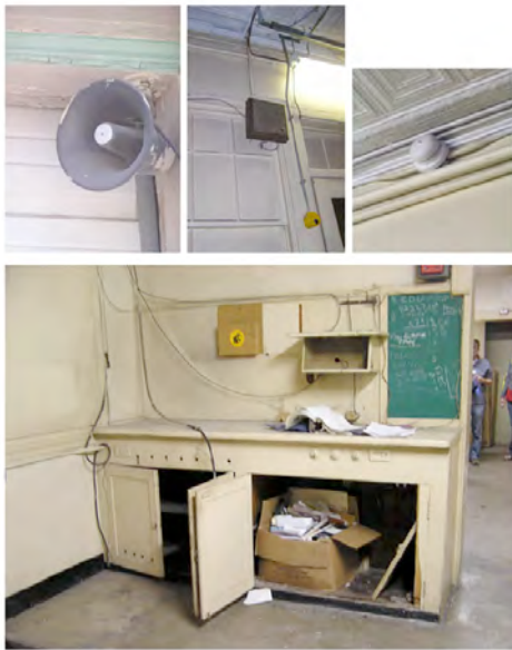
Figure 13: Alarm systems and joker stand area, Fire Station No. 11.
