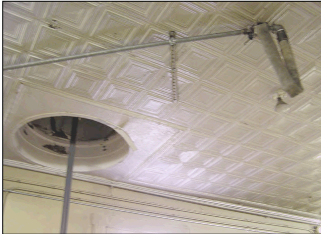
Figure 22: A pressed tin ceiling exists in the first floor apparatus bays, entry/joker stand and kitchen areas. This ceiling appears to be part of the first build because all subsequent alterations were modest, utilitarian improvements.
