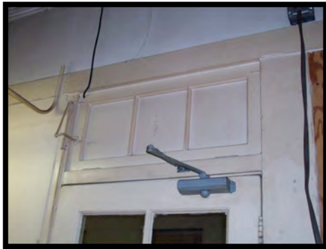
Figure 64: Doors on first level shall have working door closers
