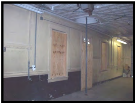
Figure 62: All doors on first level shall be verified at 3'-0" for accessibility. If door does not have clear width of 3'-0" then it shall be replaced or made non-public.
