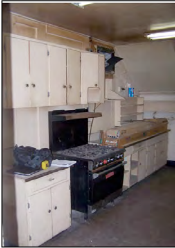
Figure 18: Current cabinetry does not appear to be part of the first build, but further investigation is needed.
