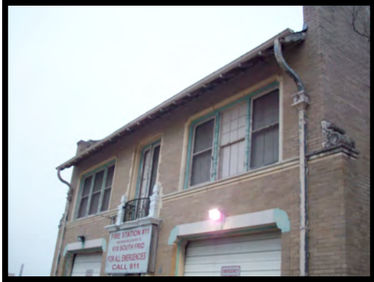
Figure 78: The existing roof decking, walls and windows will remain on the building and be reused.
