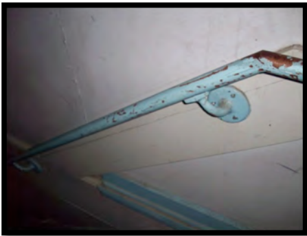
Figure 69: Handrails at stairs shall be verified with 4.26.2 and shall have proper gripping surface. If current handrails do not meet requirements they shall be replaced with new.
