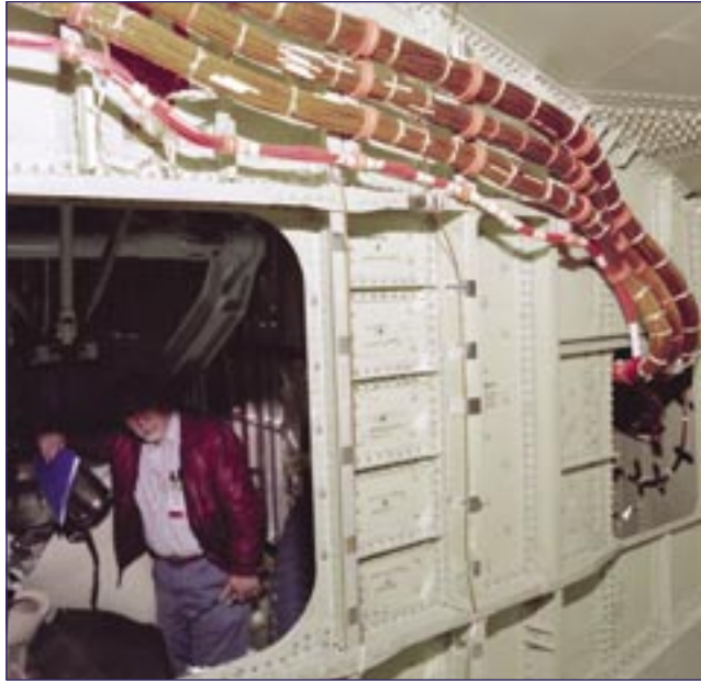
Figure 4.2-3. Typical wiring bundle inside Orbiter wing.
