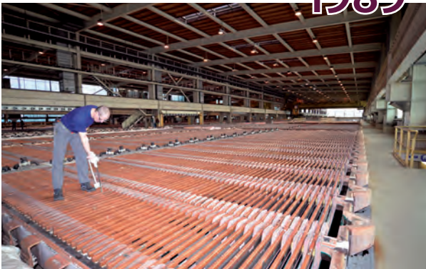
Commissioning of the tankhouse Werk Ost (ELWO)
