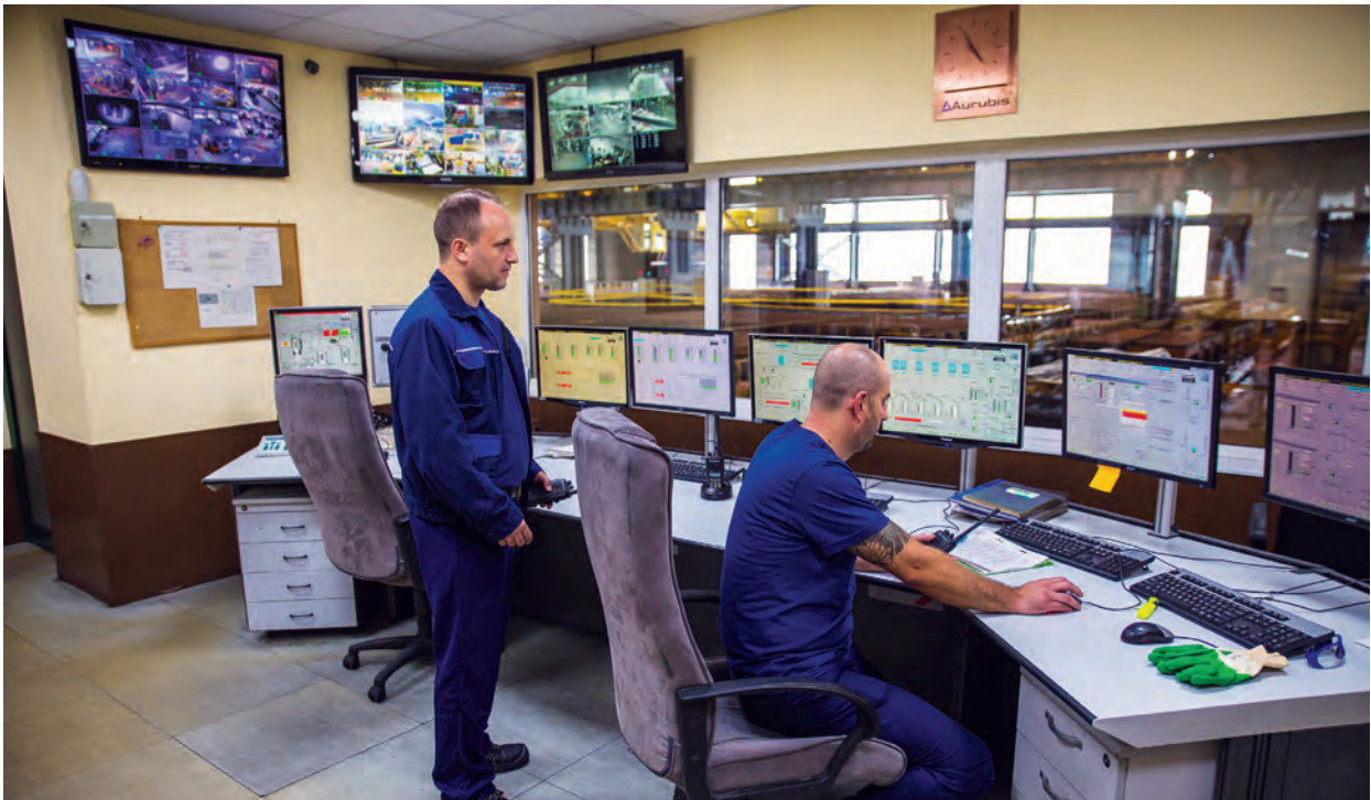
Digitally supported control and monitoring of the new tankhouse at Pirdop.
