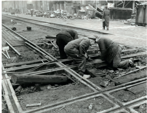
Repairing road damage at a railway crossing on the plant's northern bank in November 1944.
