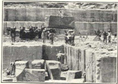
View showing a small section of "Dark Hollow"—one of the many famous quarries owned by Indiana Limestone Company.
