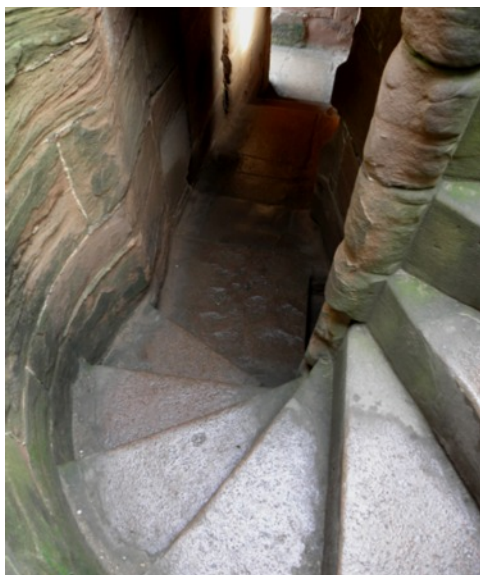
Fig 56. Kenilworth Castle - The Strong Tower. Narrow ACW stairs (0.83m) linking the room to two strong-rooms
