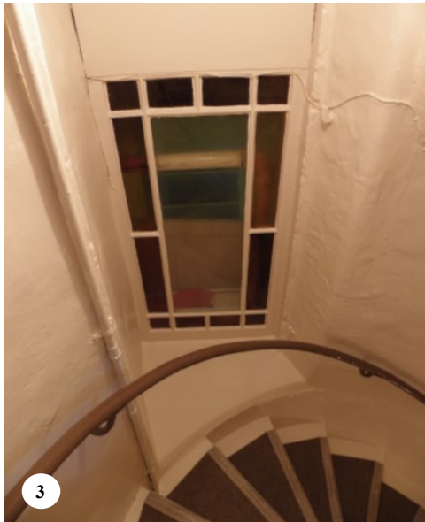
Fig. 38.3. Constable's Tower. Blocked entrance off the stairs, to the Constable's Chamber on the first floor in the adjacent main block. (See Fig. 37).
