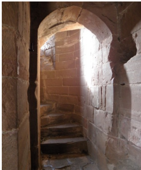
Fig 57. Kenilworth Castle - Saintlowe Tower. Narrow and steep ACW (0.83m, riser height 24 cms) stairs.
