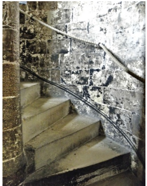
Fig. 11. Norwich Castle. ACW stair in the SE corner buttress at ground floor level. Stair treads here are modern replacements but some originals do exist.
