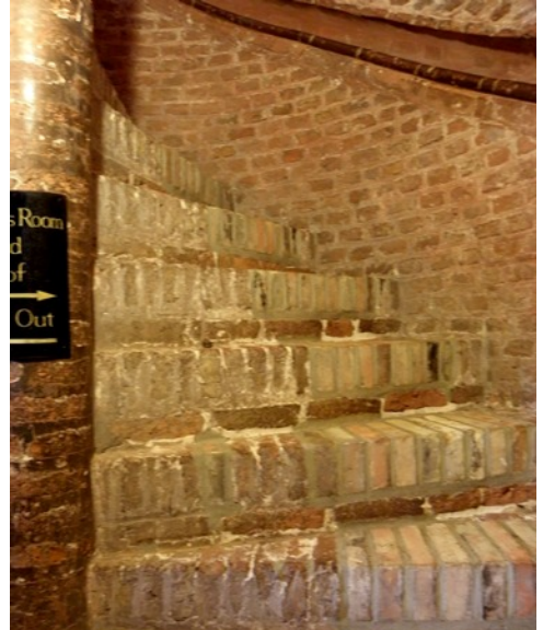
Fig. 81. Oxburgh Hall, c. 1482. The ACW newel stair in the west gatehouse turret.
