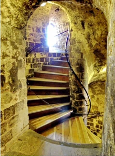
Fig. 6. The White Tower. Upper floor showing the start of the principal vaulted CW stair in the NE corner.
