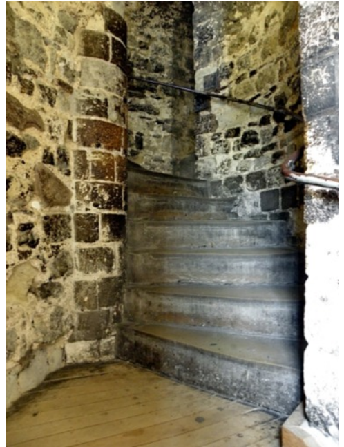
Above: Fig. 7. Upper floor access showing the secondary anticlockwise ACW stair in the NW corner.
