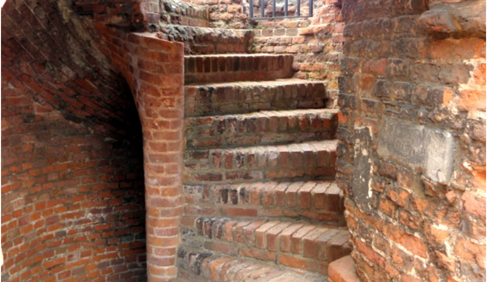
Fig. 77. Kirby Muxloe Castle, c. 1480-83. ACW stair in the gatehouse. Note: No brick moulded handrail. Stair/tread width 1.18m, Riser height 21 cms.
