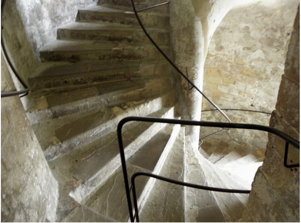
Fig. 80. Dover Castle. Great Tower NE stair turret. A view of the clockwise newel rising from the basement.
