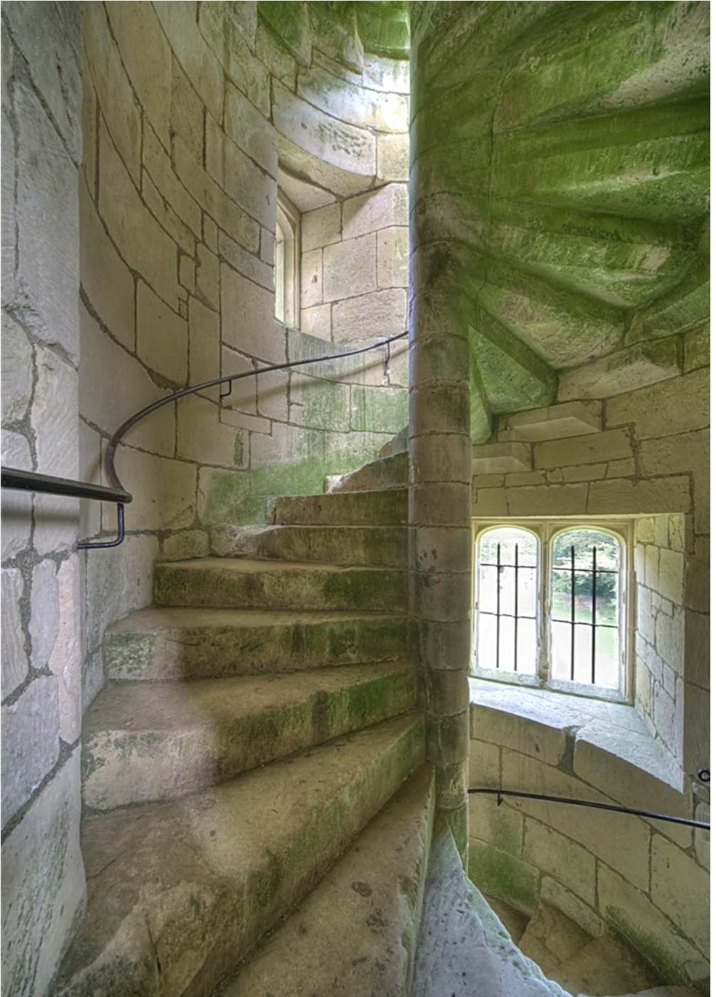
Fig. 69. Old Wardour Castle. The CW spiral stairs from the Great Hall to lodgings on the second and third floors., highlighting the quality of the stonework, the chamfered undersides of the winders and chamfered corbels inserted into the containing wall for the cut-slabs to rest on. An unusual feature in English castles.
