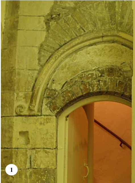
Fig. 38.1 Castle, Constable's Tower. Hoodmould over the entrance to the ACW spiral stair with unusual spiral finial or volute stop (probably added later). The hoodmould might indicate that this was once an external door, later internalised in a second phase.
