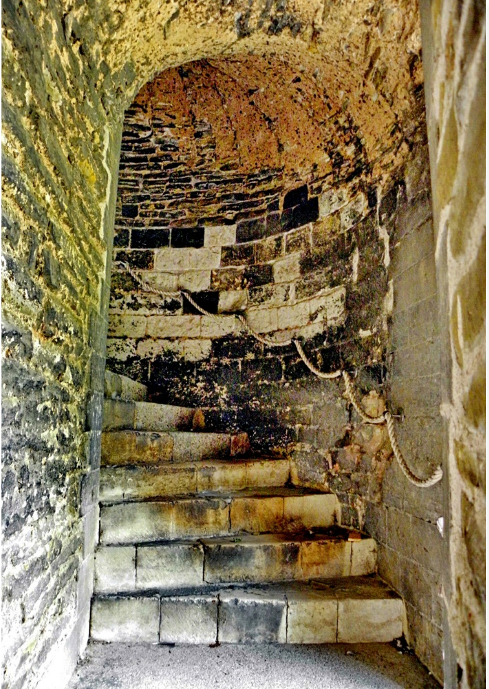
Newark Castle. Gatehouse, c. 1130-40. The wide anticlockwise spiral stair rising to the audience chamber over gatehouse passage.
