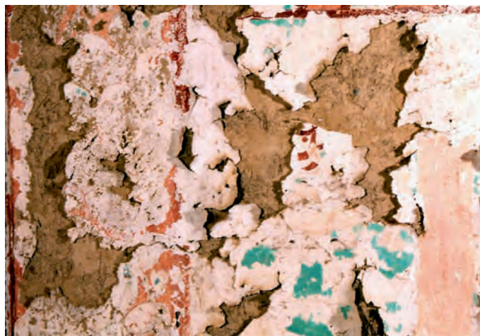
FIGURE 1 Plaster disruption of wall painting in cave 26, Mogao Grottoes, Dunhuang.
