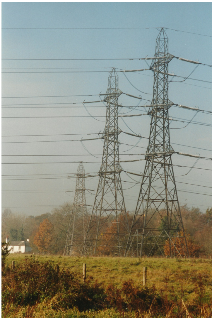
High voltage electricity transmission lines at Weybridge.
