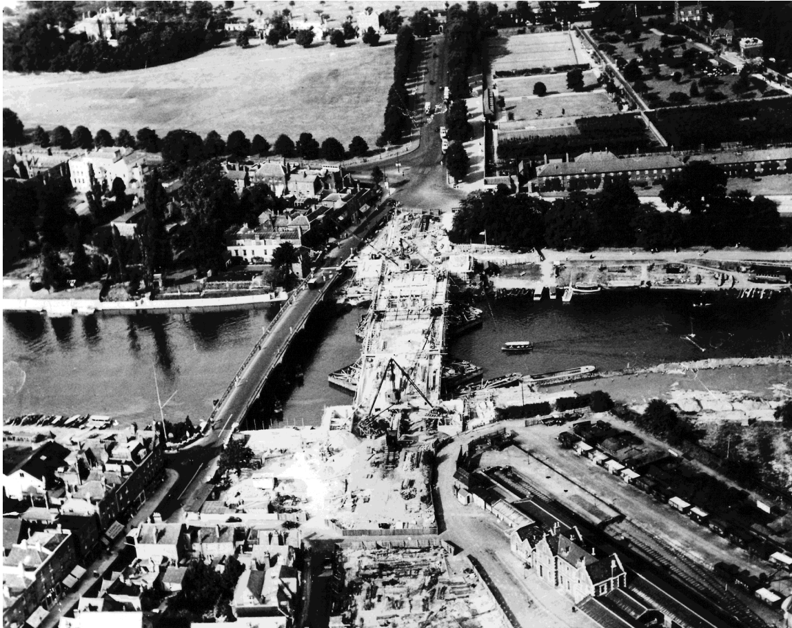
Hampton Court Bridge, architect Sir Edwin Lutyens, under construction by Surrey County Council. The bridge opened in 1933. Surrey History Centre.
