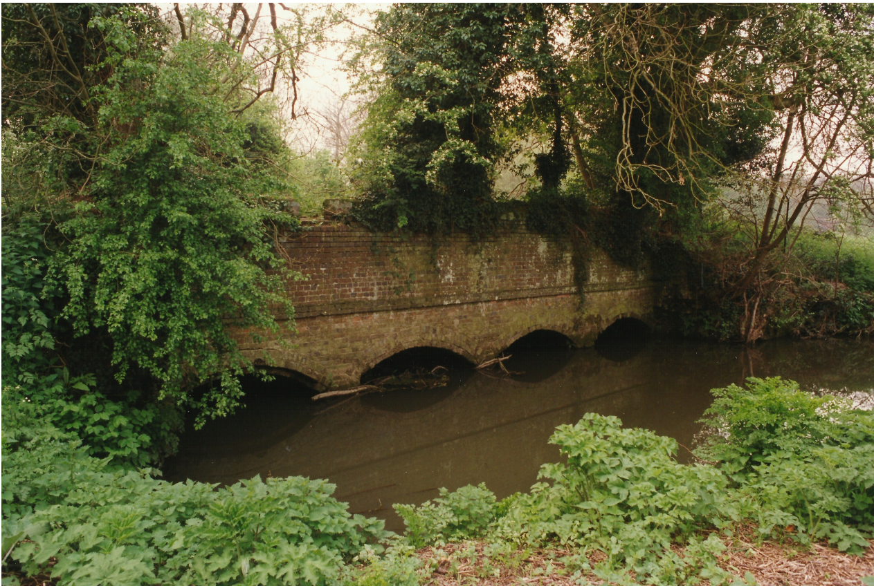
Gosden Common aqueduct carrying the Wey and Arun Canal over the Bramley Brook.
