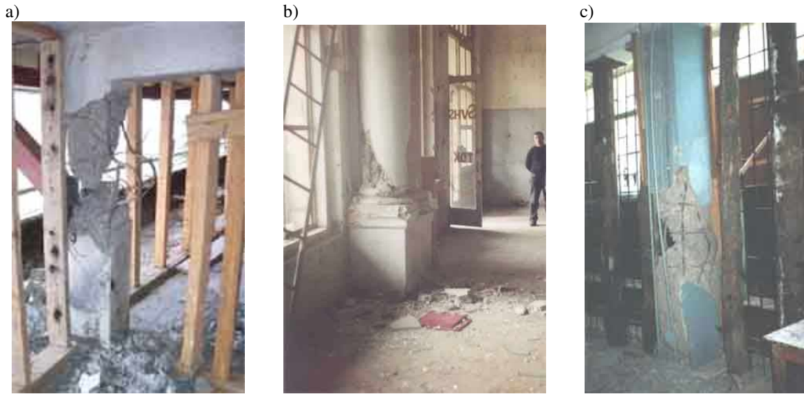
Fig. 3. Damage of columns. Inst. of Mathematics (a); Residential building in Kostava str. (b); Column of first RC floor of large-block building in Nadzaladevi District (c).
