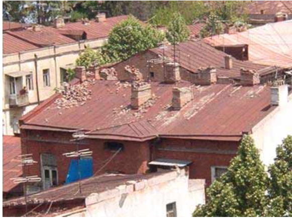
Fig. 7. Failed chimneys in Chugureti District
