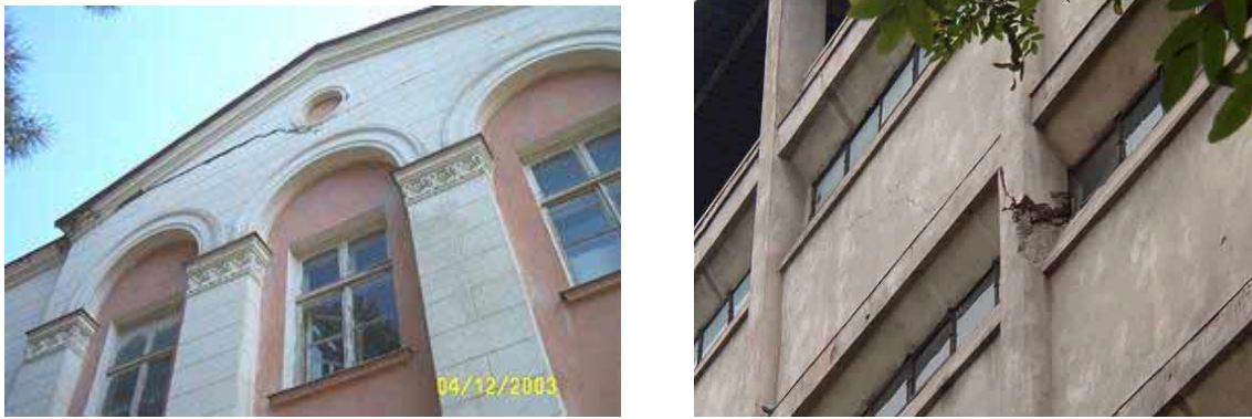
Fig. 4. Damaged brick building of hospital, A.Kazbegi str (left); Damaged column. State historical museum (right).
