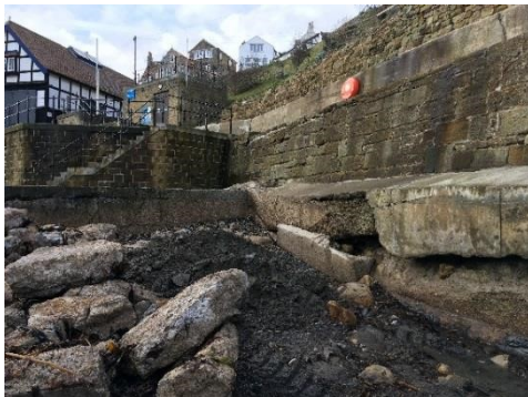
Runswick: Damage to existing sea wall
