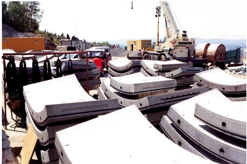
Depot for the prefabricated concrete segments for the final lining on the construction site of the Ginori service tunnel driven by TBM
