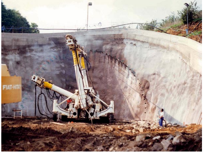
Colli Albani Tunnel. Horizontal jet-grouting to improve the ground for the South portal
