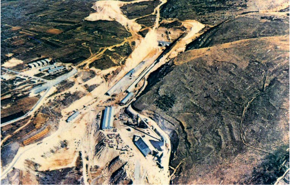
Aerial view of the construction site for the portal on the Assergi side of the Gran Sasso Tunnel
