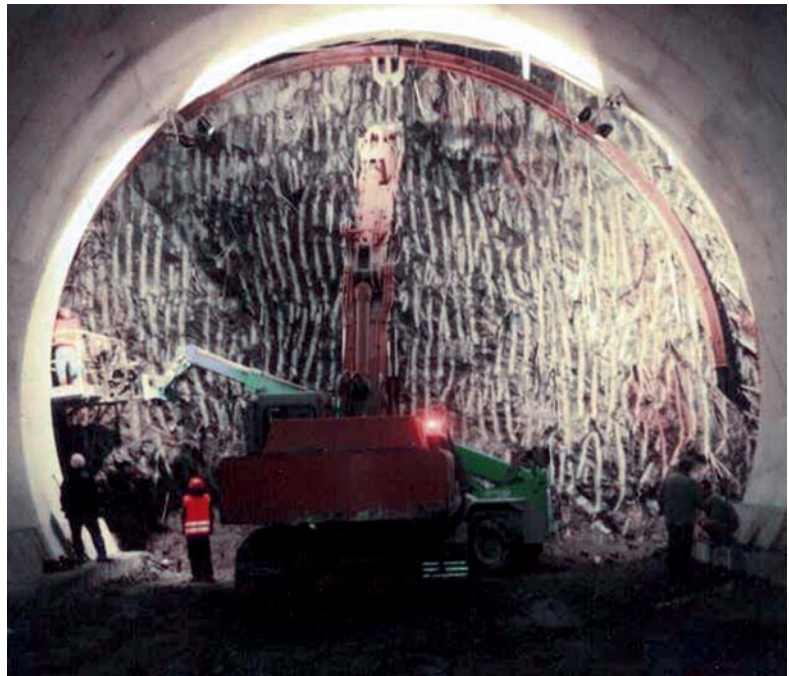
Colle Pece Tunnel. Positioning a steel rib. Ground: scaly clays, overburden: 25 m
