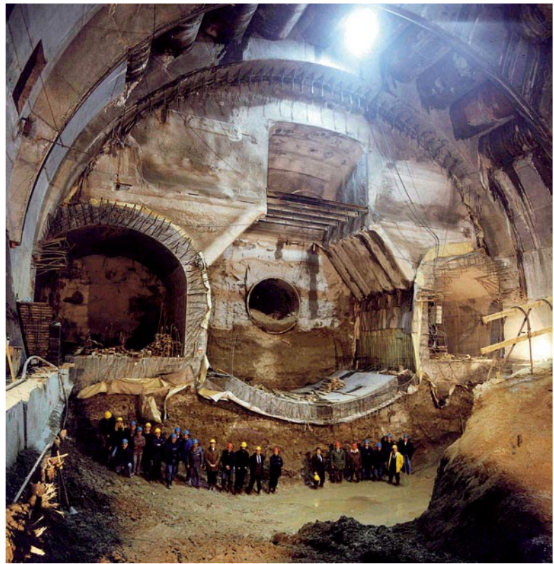
Fig. D.6 Venezia Station on the Milan urban link railway line: the full cross section
