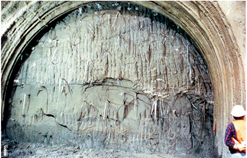
Vaglia Tunnel. View of the face reinforced using fibre glass structural elements while tunnelling through the Clays of the Mugello basin (overburden: ~ 15 m)
