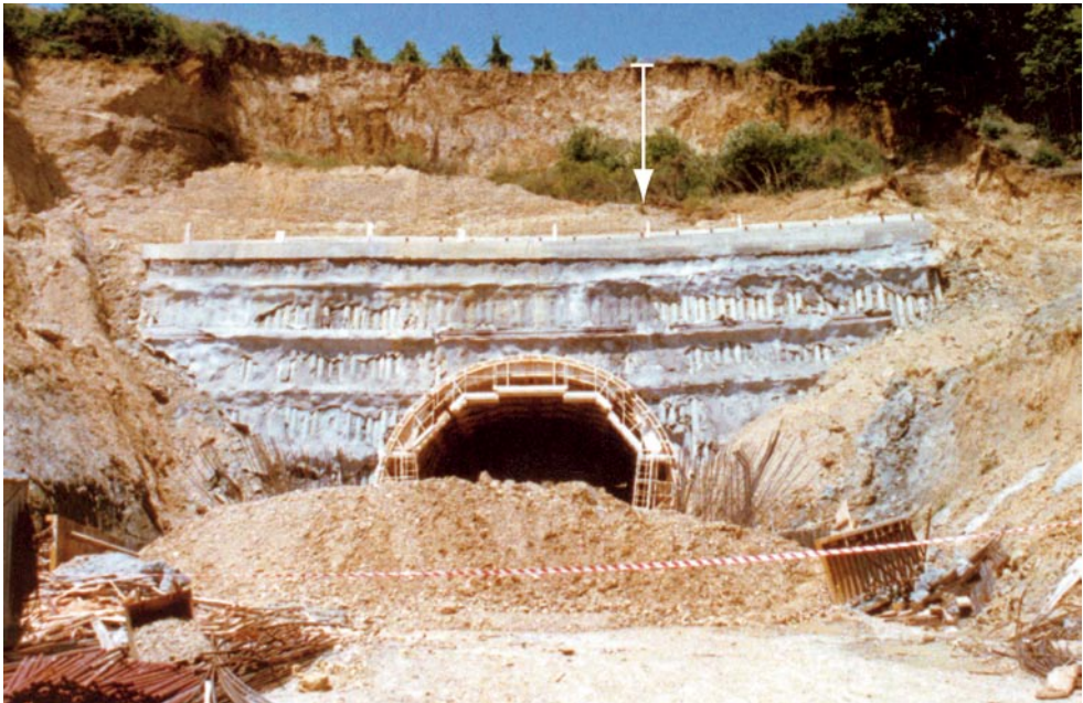
The same portal as the one above, after it had collapsed because of the decompression induced in the slope
