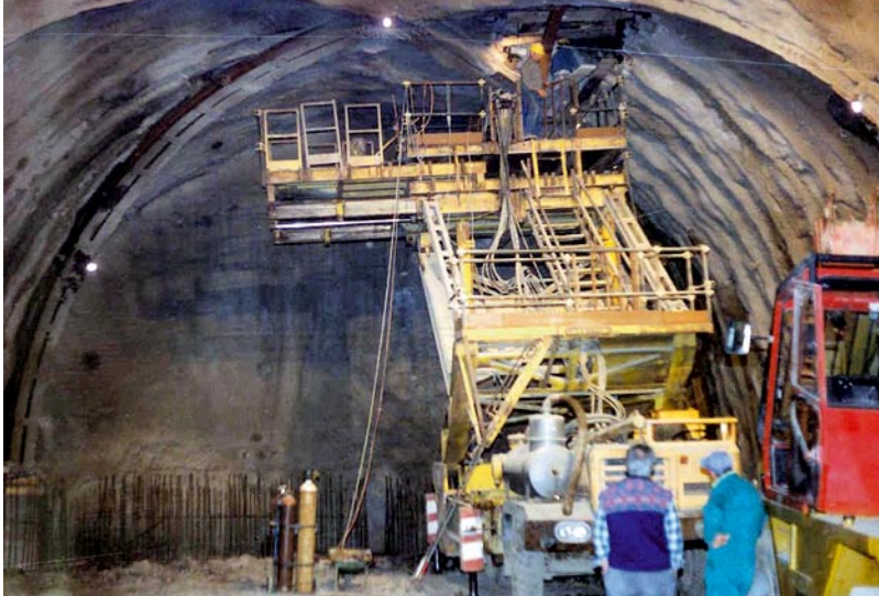
Colli Albani Tunnel. The junction with the south access tunnel, ground: vulcanites, overburden: ~ 40 m
