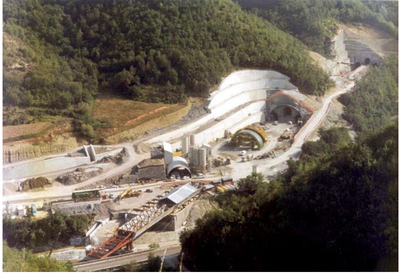
Firezuola Tunnel. View of the works for the construction of the S. Pellegrino chamber at the North portal (ground: Marly-Sandstone formation)
