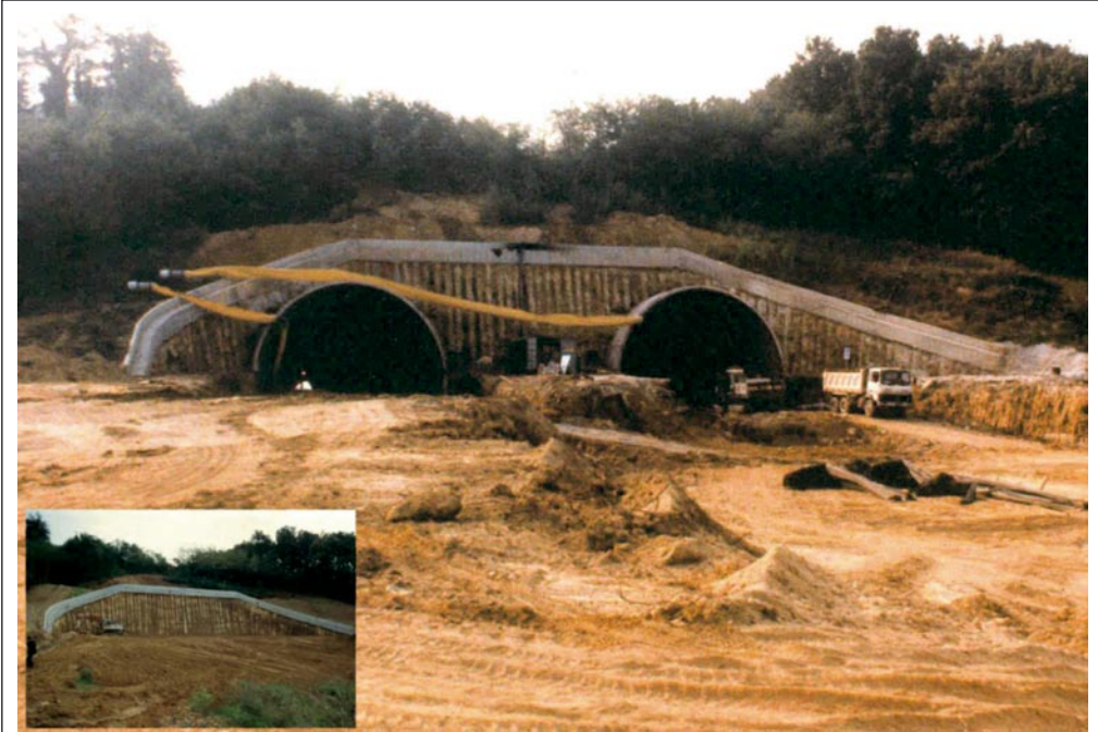
Malenchini Tunnel (Livorno-Civitavecchia motorway): North portal built by first placing a shell of ground improved by means of jet-grouting
