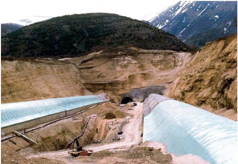
The Gran Sasso Tunnel, portal on the Assergi side: the depth of the cut made in the slope using conventional methods for the portal of the tunnel certainly makes an impression
