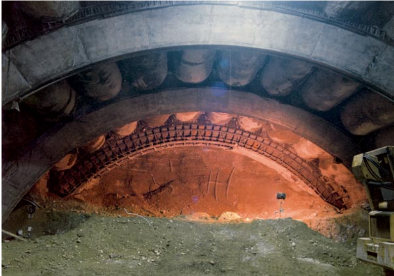
Venezia Station on the Milan urban link railway line: excavation of the station tunnel under the protection of the cellular arch already constructed. Note the presence of an arch with the formwork not yet removed
