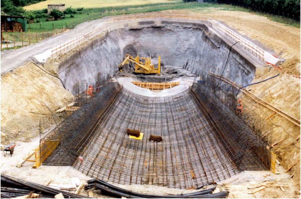
Pianoro Tunnel (new high speed/capacity railway line between Bologna and Florence): work in progress on the southern portal of the tunnel
