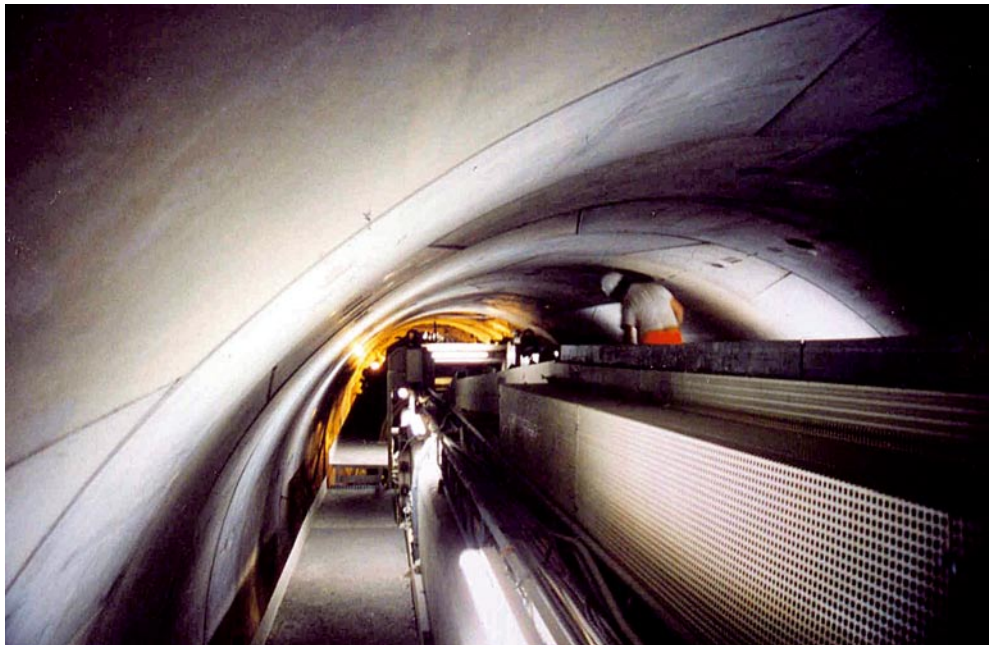
Ginori service tunnel: the "tail" of the TBM inside the tunnel already lined
