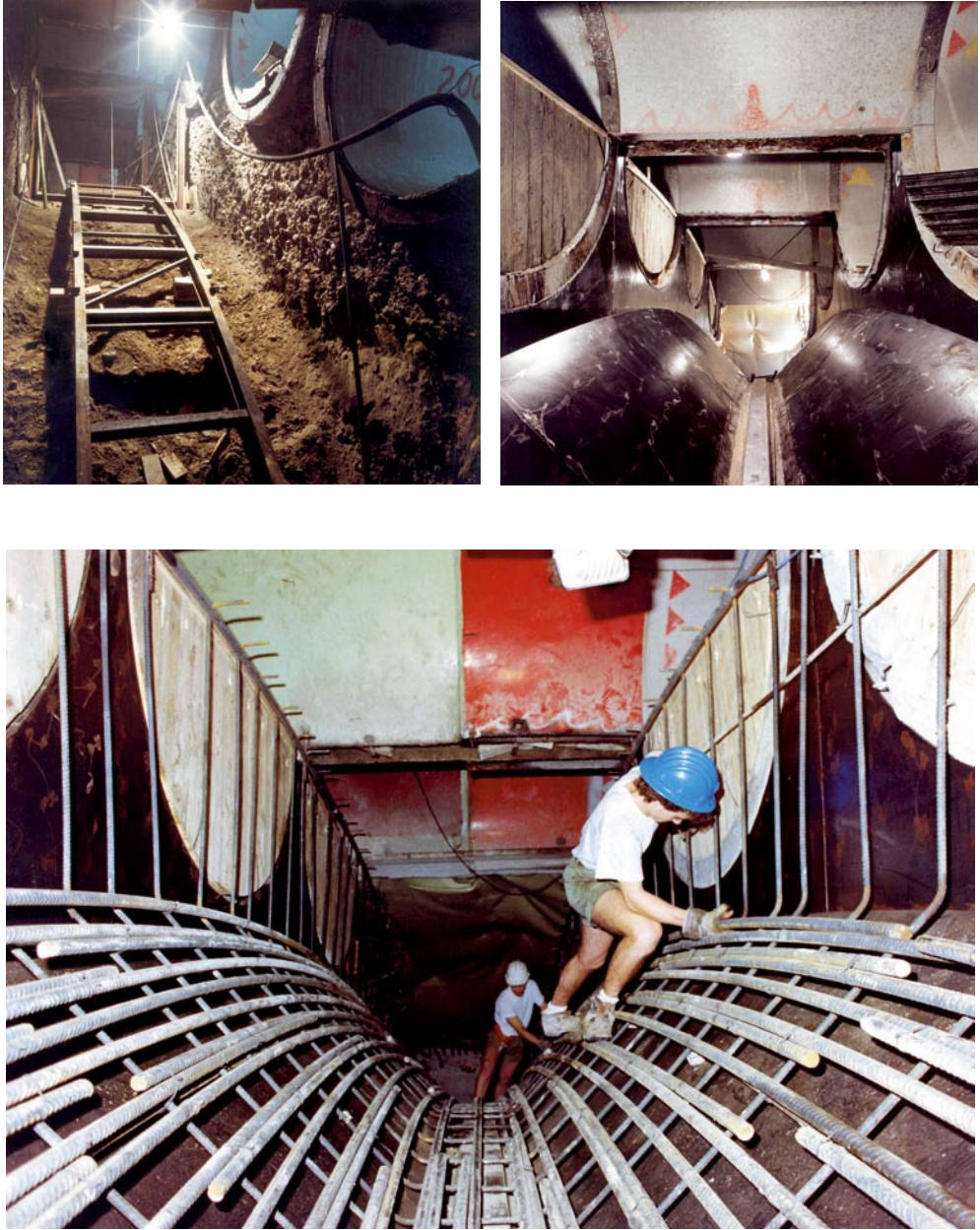
Venezia Station on the Milan urban link railway line: stages for the construction of the arches inside the transverse drifts
