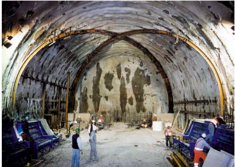
S. Giorgio access tunnel. Construction of the junction with the Firenzuola running tunnel (ground: Clays of the Mugello Basin, overburden: ~ 30 m)
