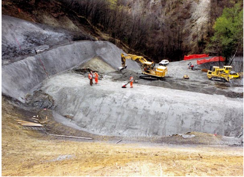
Sadurano Tunnel (high speed/capacity Bologna-Florence railway line): view of the 'sprayed' crown of the future bored tunnel
