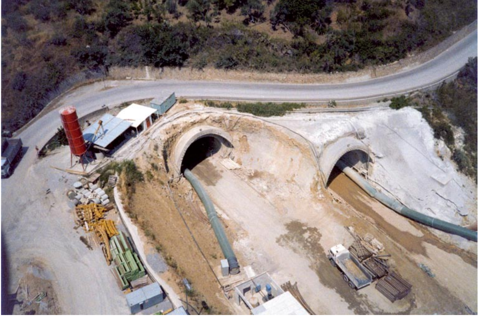
S. Elia Tunnel (Messina-Palermo motorway): portal on the Messina side under construction under the provincial Cefalù-Gibilmanna road
