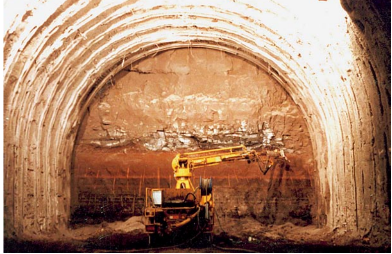
Colli Albani Tunnel. Work to reinforce the core-face, ground: vulcanites, overburden: ~ 30 m
