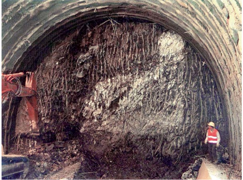
Colle Pece Tunnel. Face reinforced with fibre glass structural elements. Ground: scaly clays, overburden: ~ 25 m
