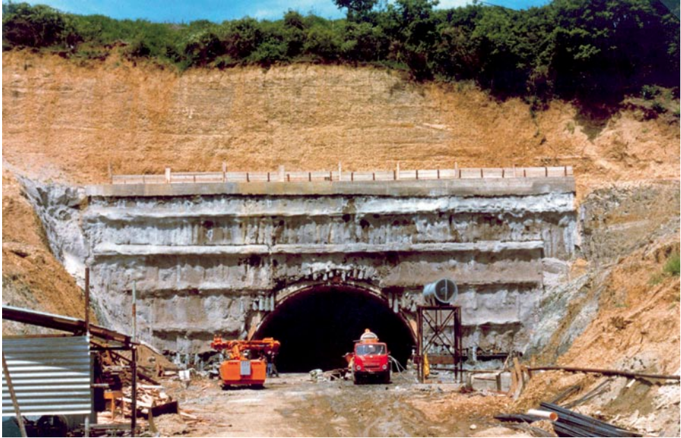
A very deep cut is made into the slope for a tunnel portal in semi-cohesive soils using conventional systems (anchored Berlin wall; overburden: twice the diameter of the tunnel)
