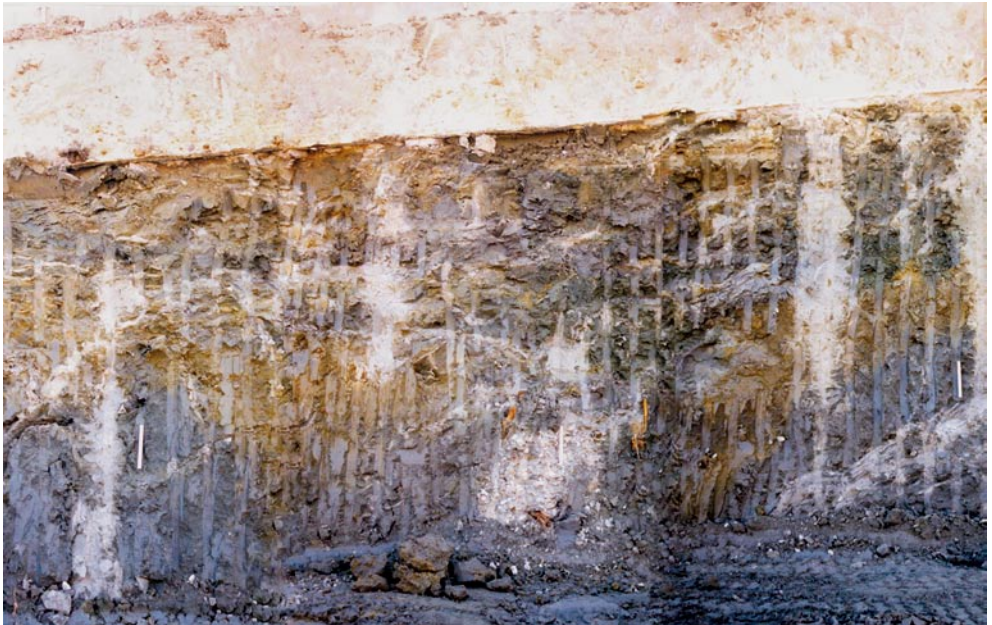
Detail of the wall of a shell of columns of ground improved by means of vertical jet-grouting
