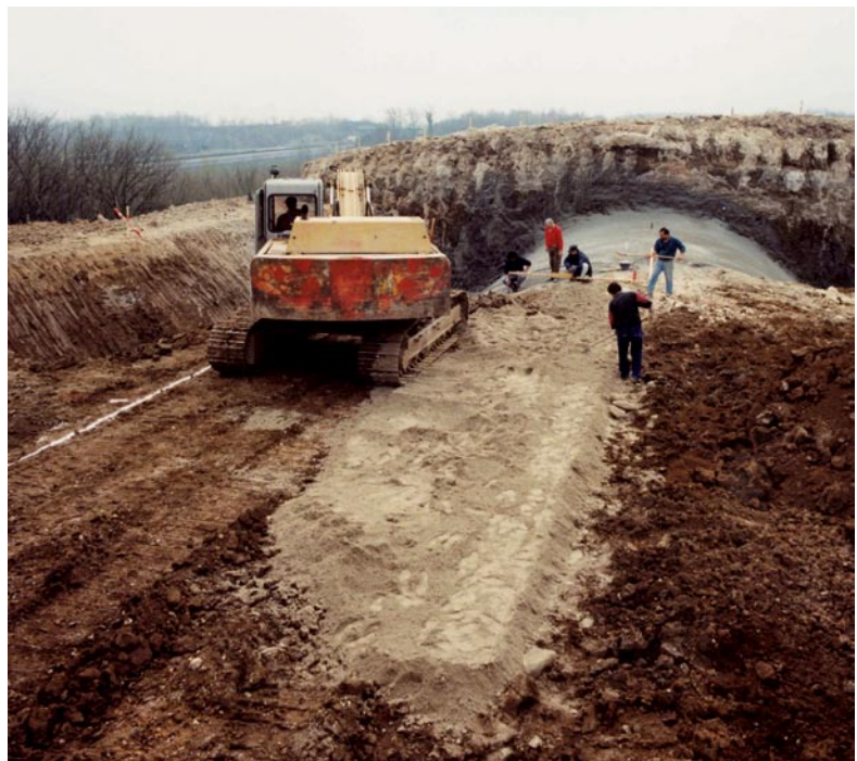
Santuario Tunnel. Treatment of the ground with lime to create Artificial Ground Overburden (A.G.O.), type of ground: pyroclastites
