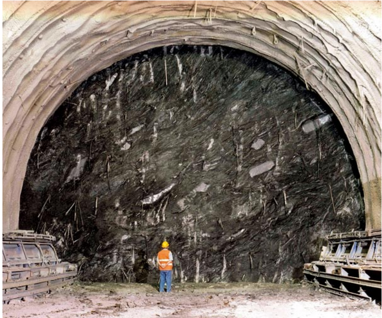
Raticosa Tunnel. Reinforcement of the core-face by means of fibre glass structural elements in the scaly clays of the Complexo Caotico (overburden: ~ 550 m)
