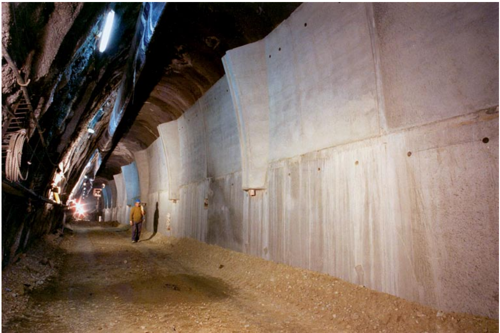
Venezia Station on the Milan urban link railway line: the construction of a sidewall in a side drift
