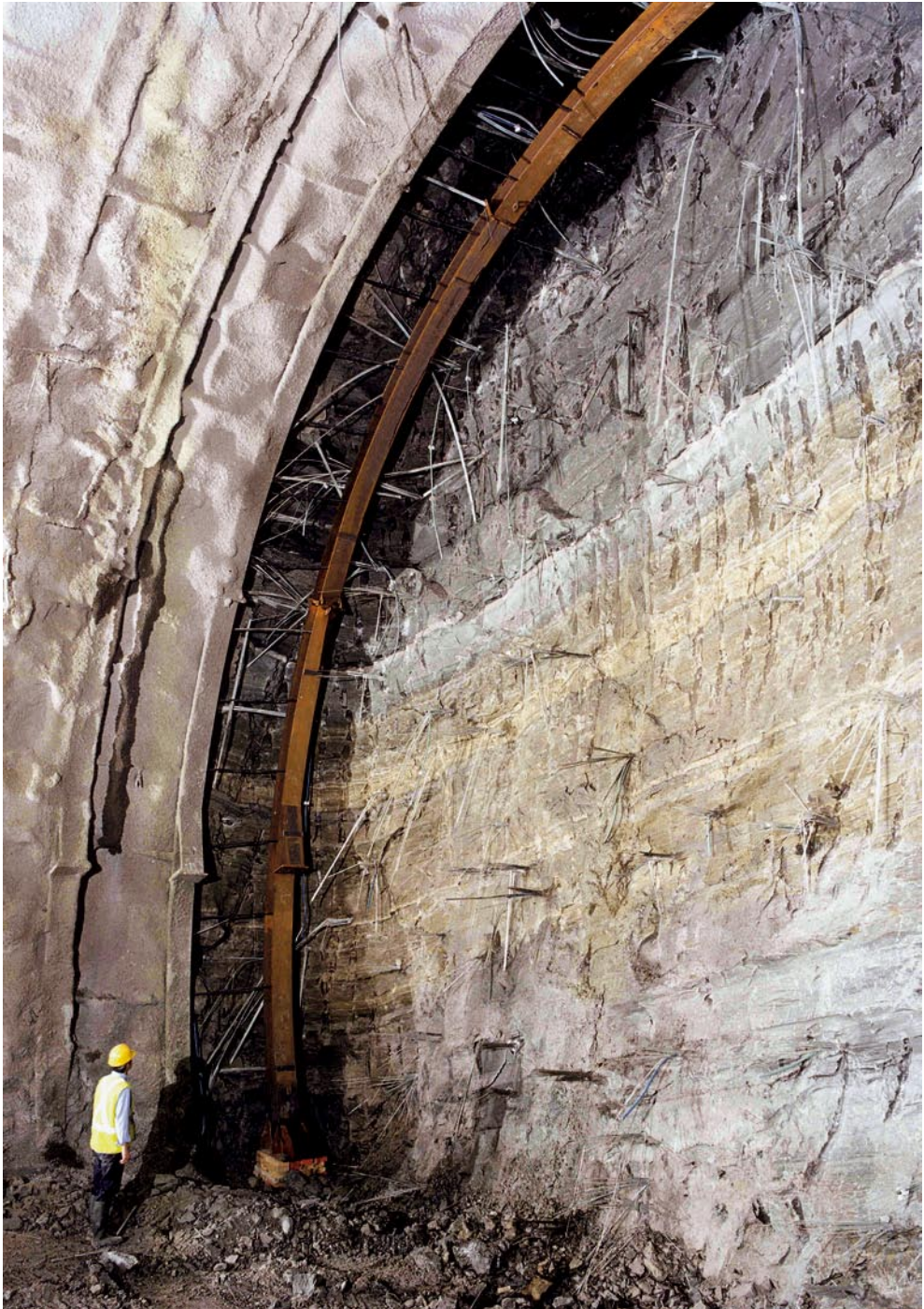
The Tartaguille tunnel: the core-face reinforced with fibre glass elements, 1997, ground: clay, max. overburden: ~ 110 m
