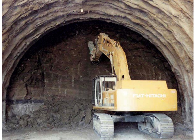
Macchia Piana Tunnel. Demolition of the core-face using a demolition hammer (ground: tuff, overburden: ~ 3 m)
