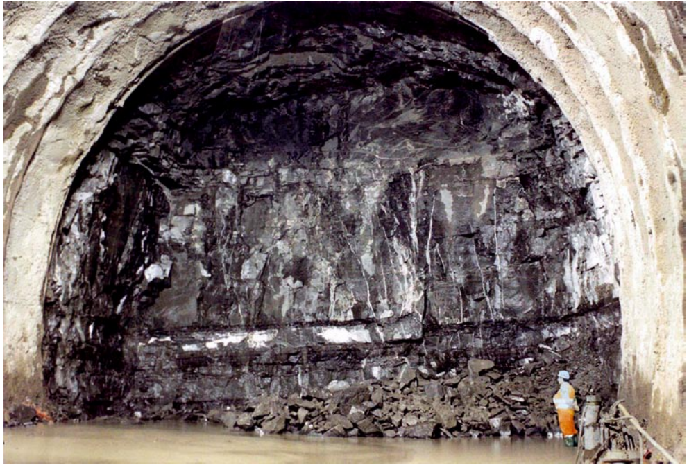
Firezuola Tunnel. View of the face while tunnelling through the Marnoso-Arenacea formation (overburden: ~ 500 m)
