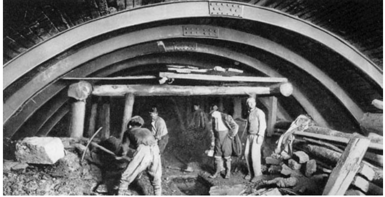
Bologna-Florence Direttissima Line, excavation of the Grand Apennine Tunnel: reinforcement in the crown with steel ribs
