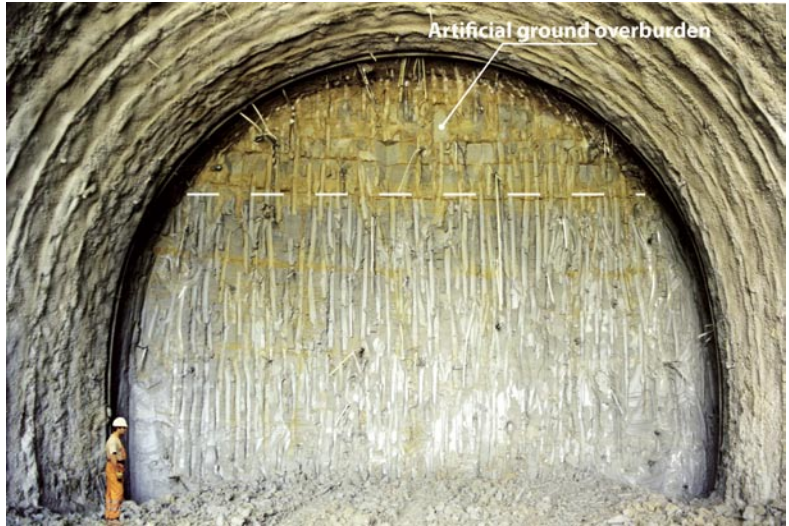
Borgo Rinzelli Tunnel: effect of stabilisation using artificial ground overburden (ground: Clays of the Mugello Basin, overburden: zero)
