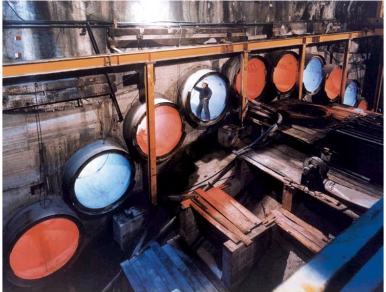
Venezia Station on the Milan urban link railway line: a view of the thrust pit after the minitunnels have been driven
