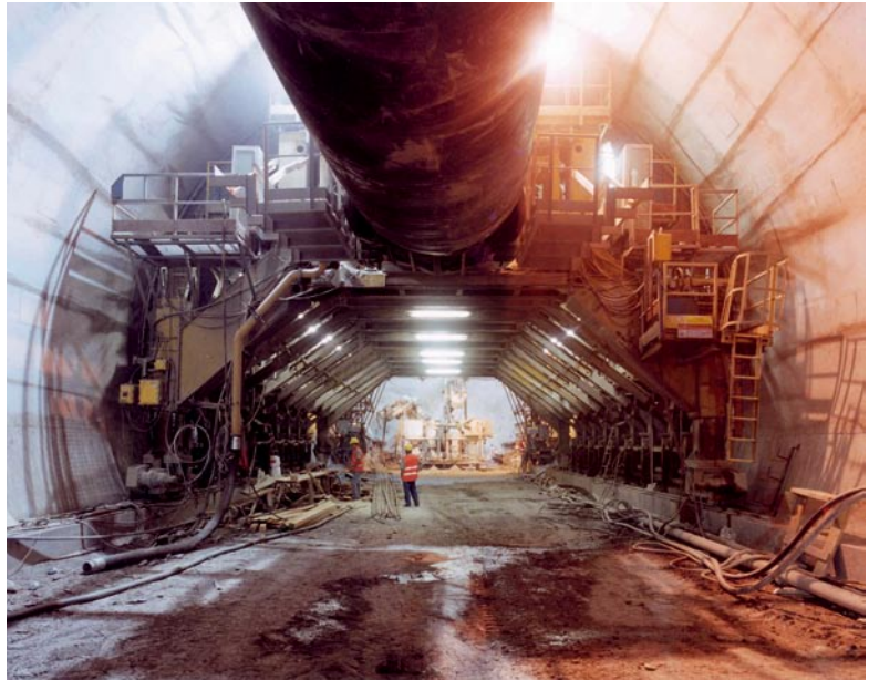
Raticosa Tunnel. Mobile formwork for casting the final lining in reinforced concrete
