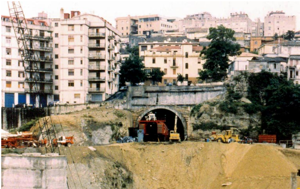
S. Giovanni Tunnel (Catanzaro ring road East): tunnel portal with diameter 14 m approx., excavation under urban buildings
