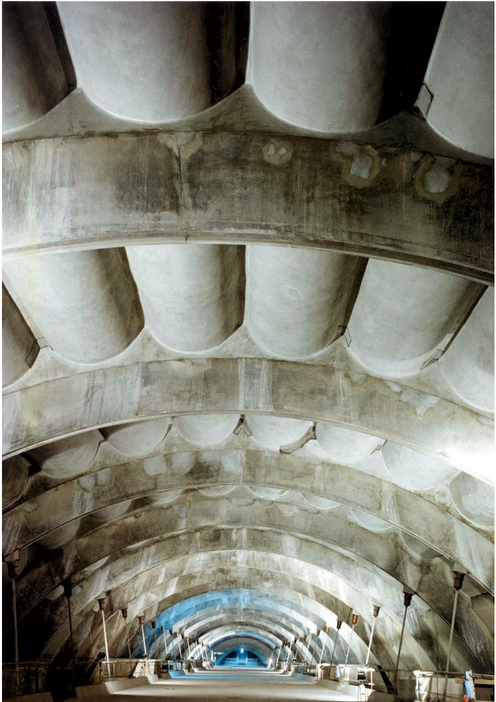
Cellular arch technology: view of the structure built for the Venezia station of the Milan urban link line (1990, ground: sand and gravel under the water table)
