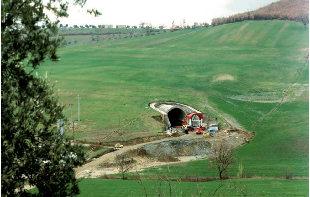
Tunnel No. 2 (Sibari-Cosenza railway line): the use of jet-grouting technology enables tunnel portals to be built in difficult grounds with full respect for natural equilibriums and for the landscape
