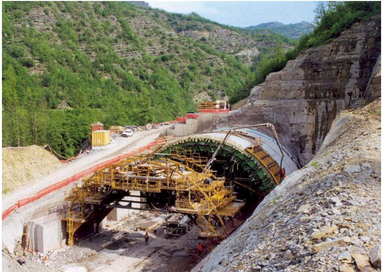
Firezuola Tunnel. Construction of the artificial tunnel of the S. Pellegrino chamber at the North portal (ground: Marly-Sandstone formation)
