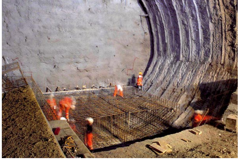
Raticosa Tunnel. Reinforcement of the tunnel invert very close to the face (ground: scaly clays of the Complesso Caotico, overburden: ~550 m)
