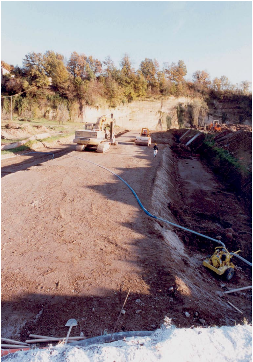
Rome-Naples high speed/capacity railway line, Piccilli 2 tunnel. Construction of the "artificial ground overburden (AGO)" in the section with no overburden, ground: pyroclastites
