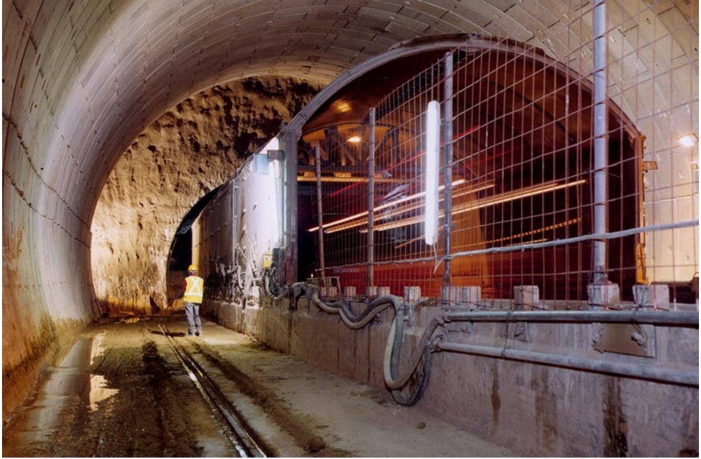
Fig. G.14 The steel shell to protect traffic. The tracks on which the machine moves can be seen at the bottom of the photo
