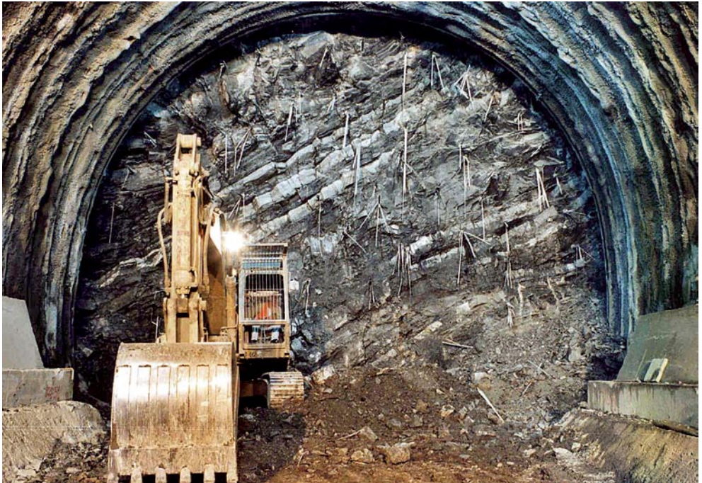
Monte Bibele Tunnel. View of the face while tunnelling through the Monghidoro Flysch, overburden: ~ 200 m)
