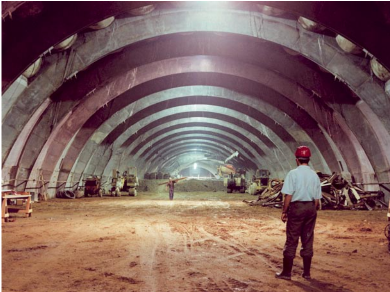
Venezia Station on the Milan urban link railway line: a view after half face excavation
