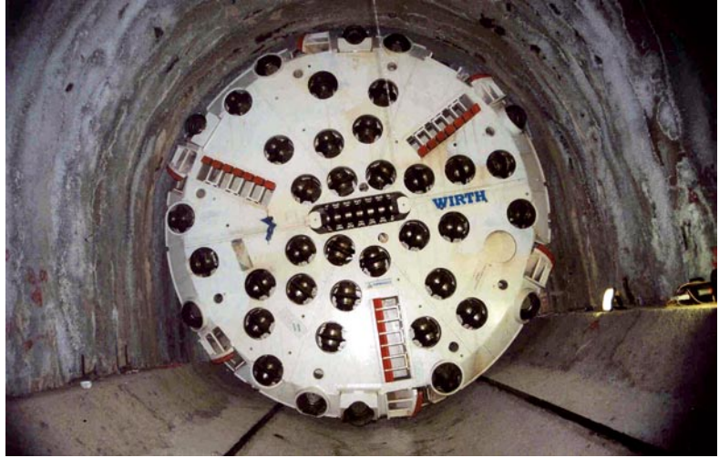
Ginori service tunnel: view of the head of the TBM during insertion in the tunnel
