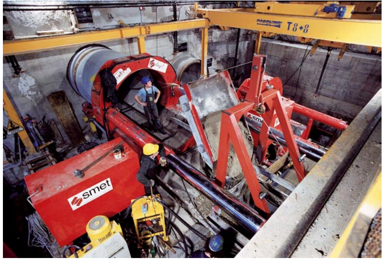
Venezia Station on the Milan urban link railway line: pipe jacking to drive minitunnels side by side around the perimeter of the roof arch of the station
