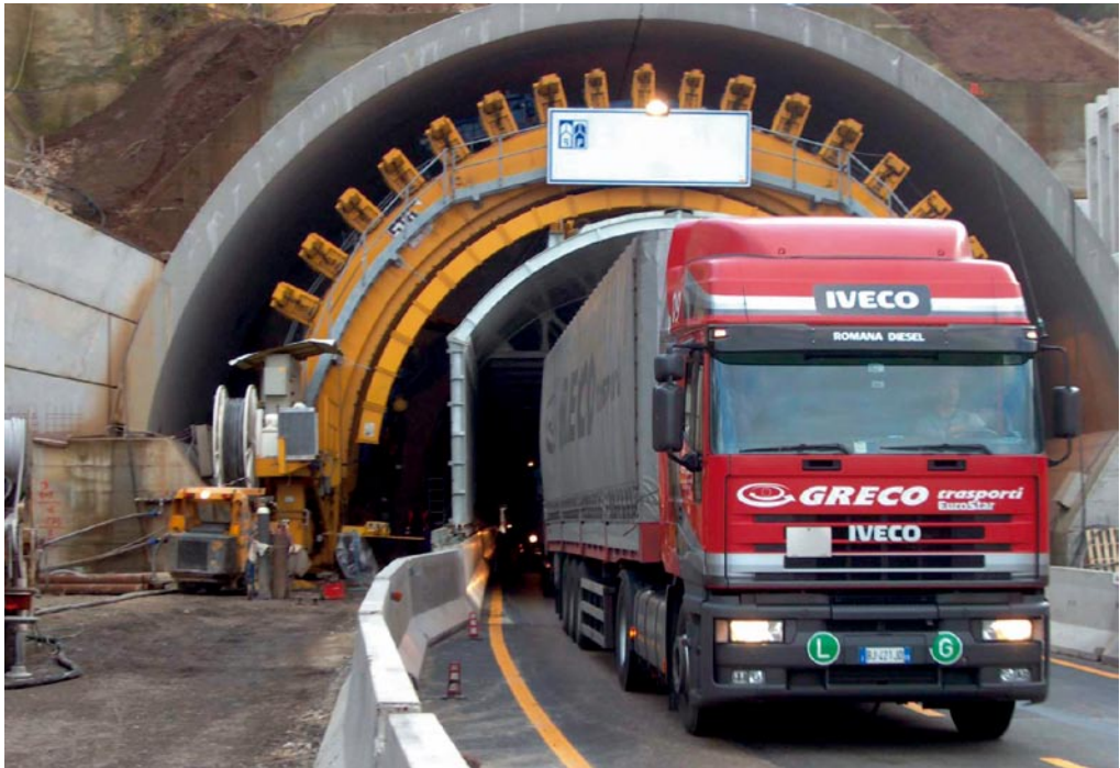
Fig. G.13 The work to widen the tunnel was performed with the motorway in service
