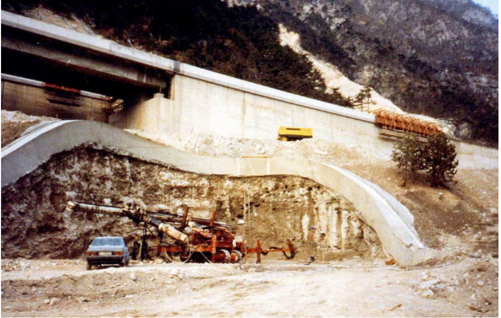
A shell of columns of ground improved by vertical jet-grouting constructed for the portal of the S. Leopoldo tunnel under the motorway embankment
