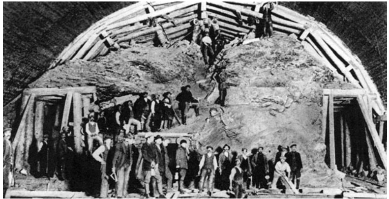
Bologna-Florence Direttissima Line, excavation of the Station chamber from the previous Grand Apennine Tunnel: steel ribs in the crown and side drifts
