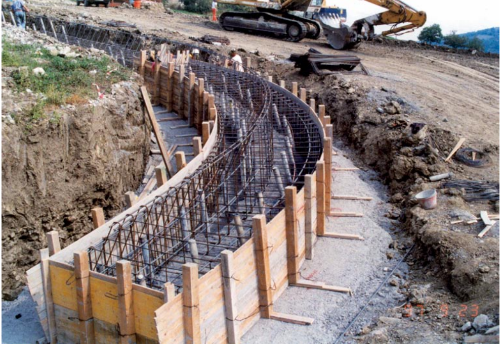
Preparation for casting the upper r.c. beam over a shell of ground improved by vertical jet-grouting
