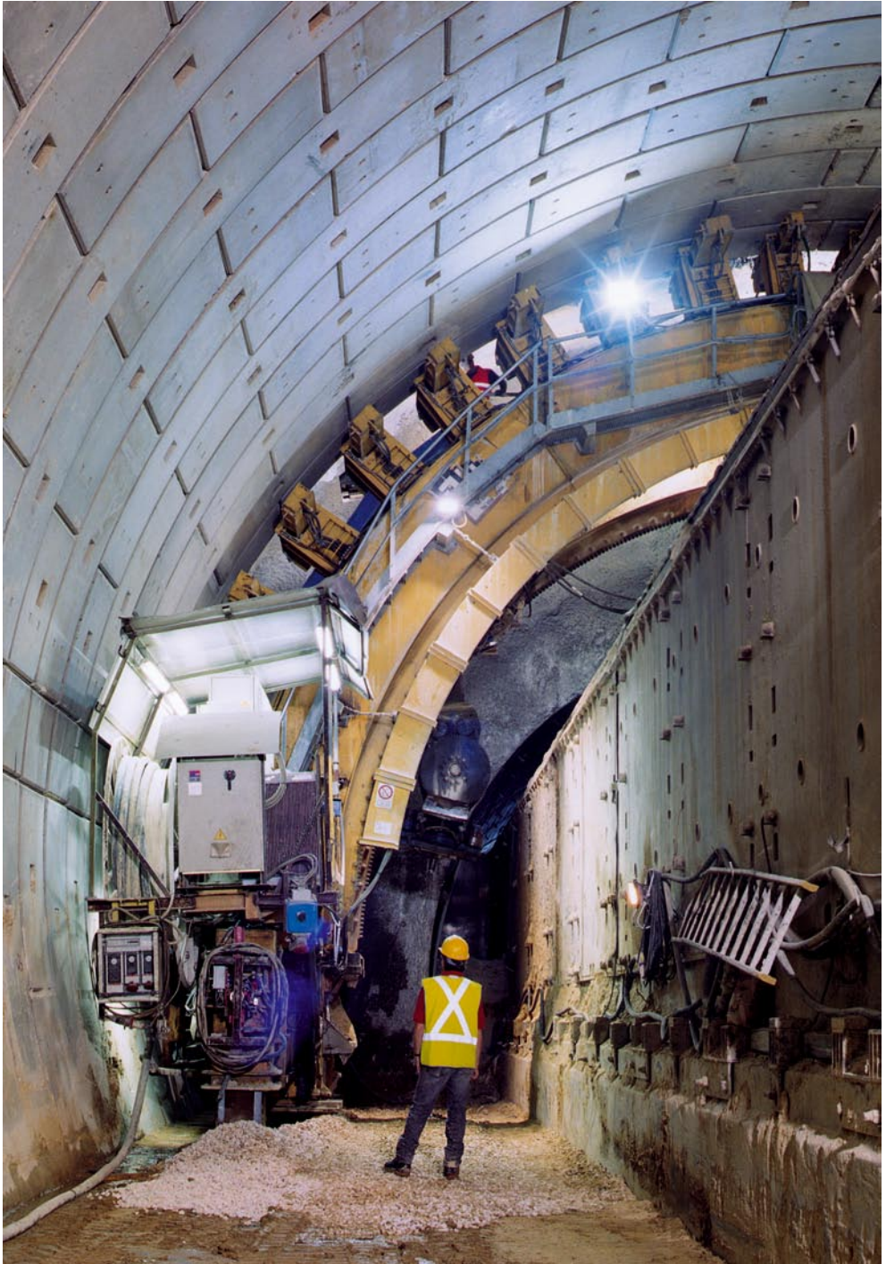
Widening of tunnels without interrupting traffic: Milan-Rome motorway, Nazzano tunnel, placing an arch of the lining constructed using prefabricated segments (2005)
