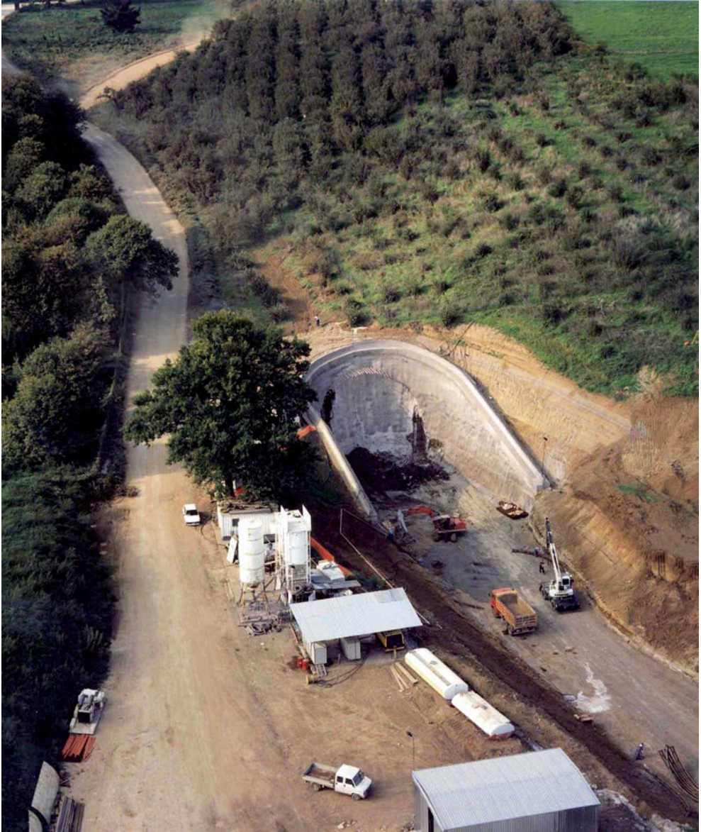
Colli Albani Tunnel (new Rome-Naples high speed railway line): aerial view of the works for the construction of the South portal of the tunnel
