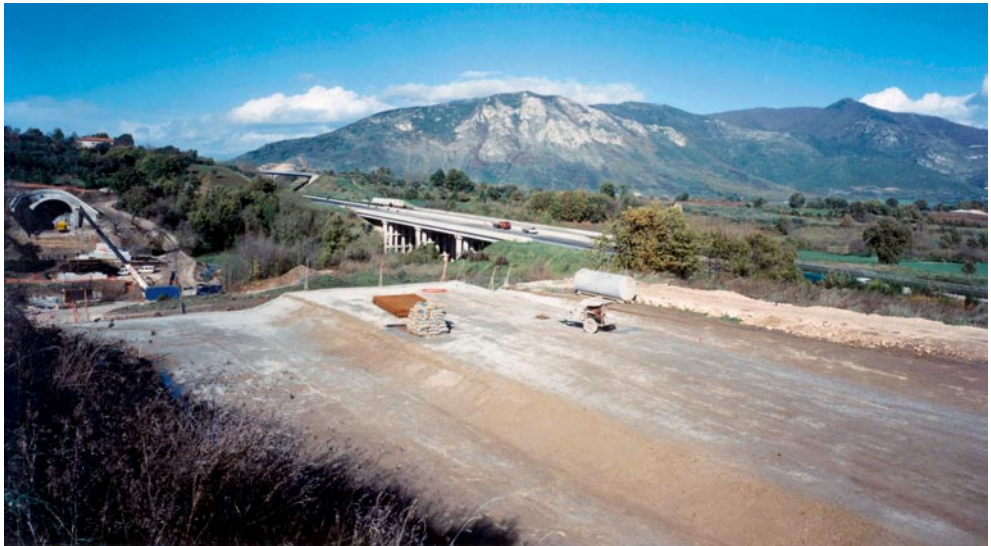
Piccilli Tunnel 1 (above) and 2 (below): two stages in the construction of the A.G.O.
