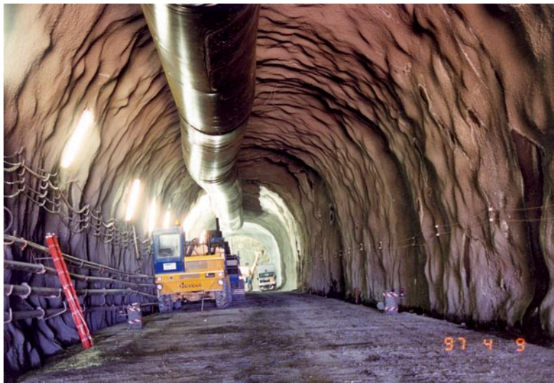
Castelvechio access tunnel. The construction of 9 tunnels on the new high speed/capacity Bologna-Florence railway line required the construction of 14 access tunnels for a total length of 9,255 m
