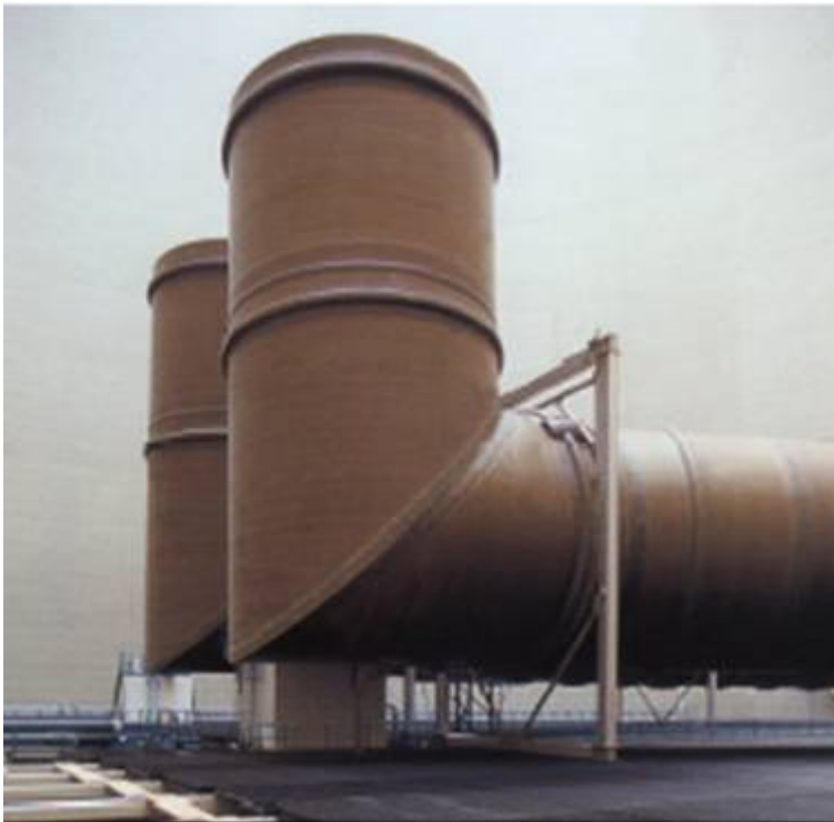
Figure 32: FGD Boxberg (Germany) – Cooling Tower Discharge
