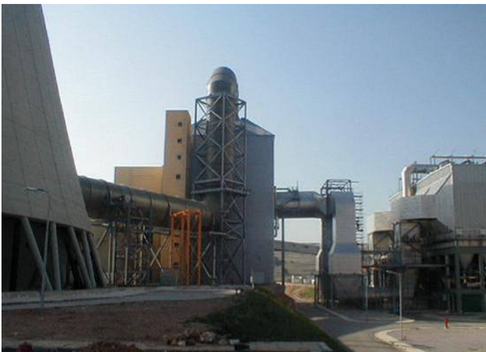
Figure 33: Cooling tower introduction of the flue gases, Florina power station, Greece
