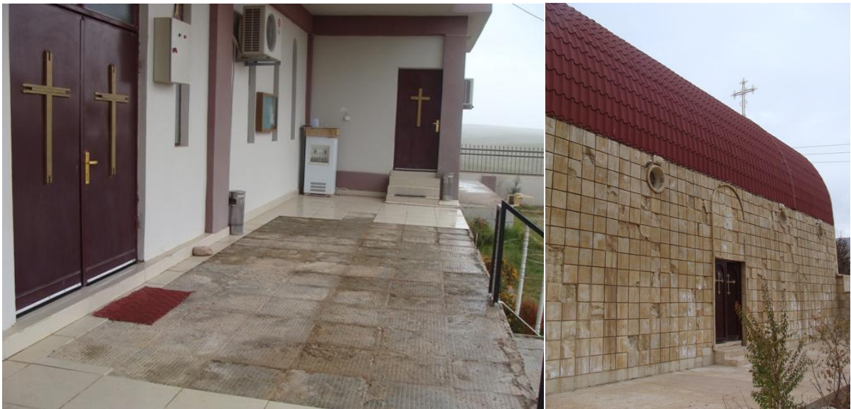
Churches by Aghajan and the KRG: St. George's Ancient Church of the East in Bakhitme (left). Not only has the paint peeled off the dome, but the floor tiles have also come loose. At St. Sawa's Assyrian Church of the East in 'Ayn-Nune (right), the marble facade has dangerously cracked and is collapsing.
