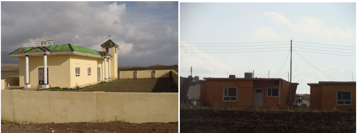
At oil-rich but impoverished Navkandala, not only have the roof tiles of the Aghajan-built church gone green (left), but many of the houses (right) are so dangerously cracked they are practically uninhabitable.
