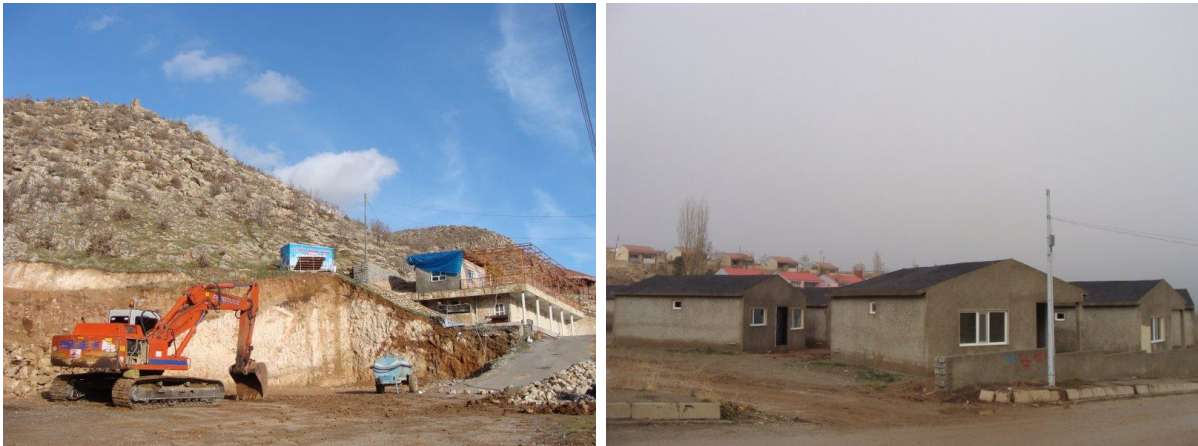
Left: Developing the touristic cave restaurant at Inishk; Right: Tourist chalets under construction at Sarsing.
