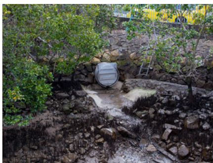
Backflow prevention device
