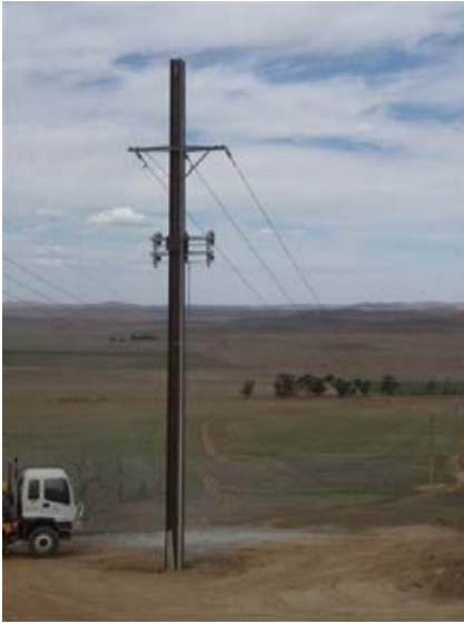
Figure 2.4 33 kV overhead feeder lines
