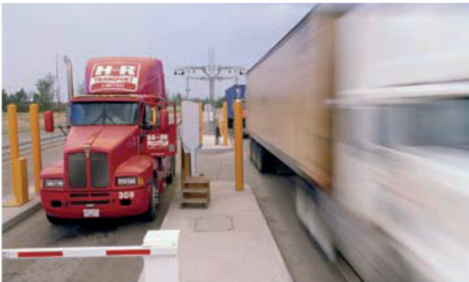
Figure 53. Automated Gate System: driver clearance post
