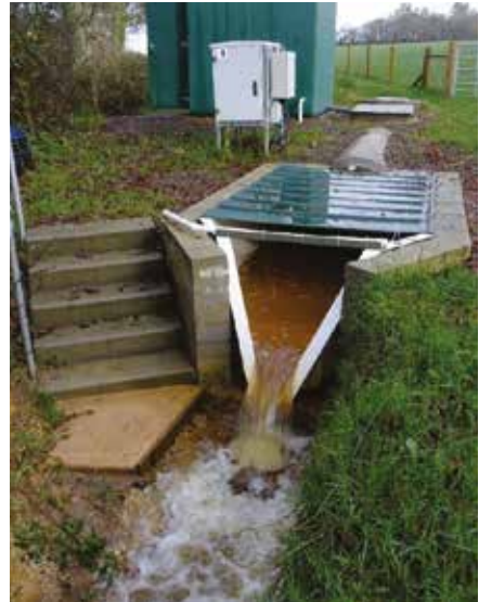
Catchment flumes and instrumentation cabin
